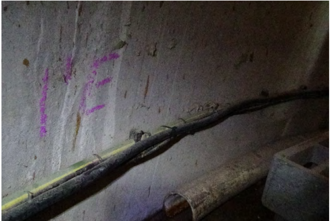
1' E—The circuit and electrical cables are properly secured to the concrete column in a tidy fashion .
