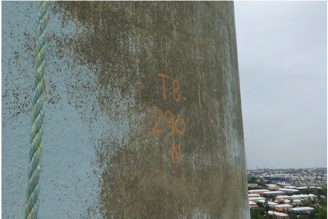
230' N—A large area of bare concrete is visible at this elevation. The remainder of the coating is weathered, the paint appears to be “washing” off the concrete rather than peeling.
