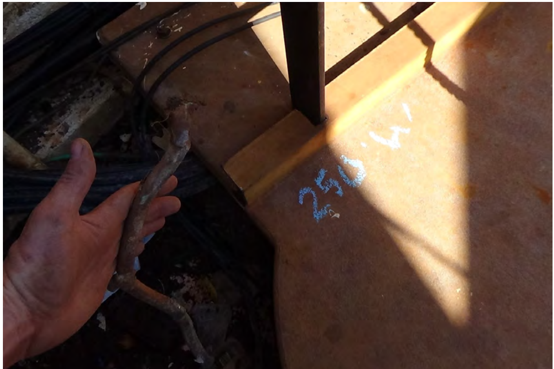
250' W—Photo taken on the roof deck shows that the ground cable connecting the liner grounds to the copper downlead has been sheared.
