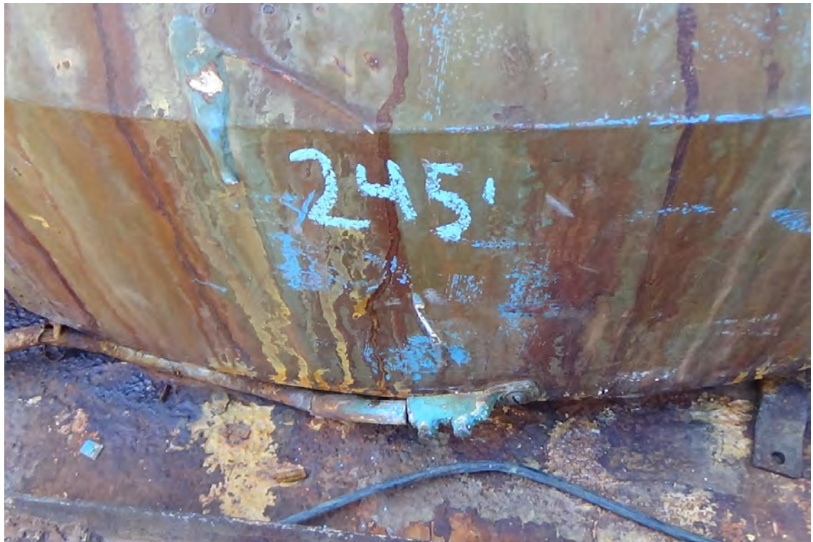
245' W—The ground connection to the skirt of flue #1 is present and intact. The same ground cable was found to be severed near the connection point to the downlead. This appears to be the only location in which the liner is grounded.
