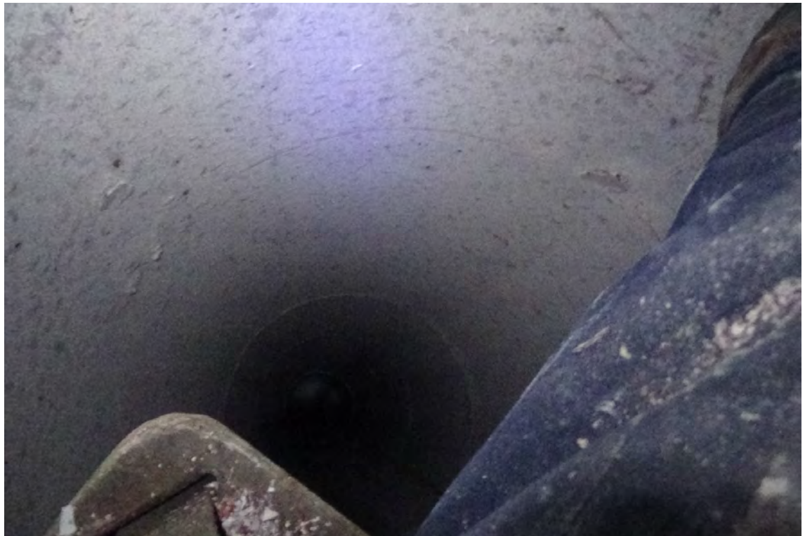
80' S/F2—View looking down the interior wall illustrates that scaling is less noticeable at lower elevations.
