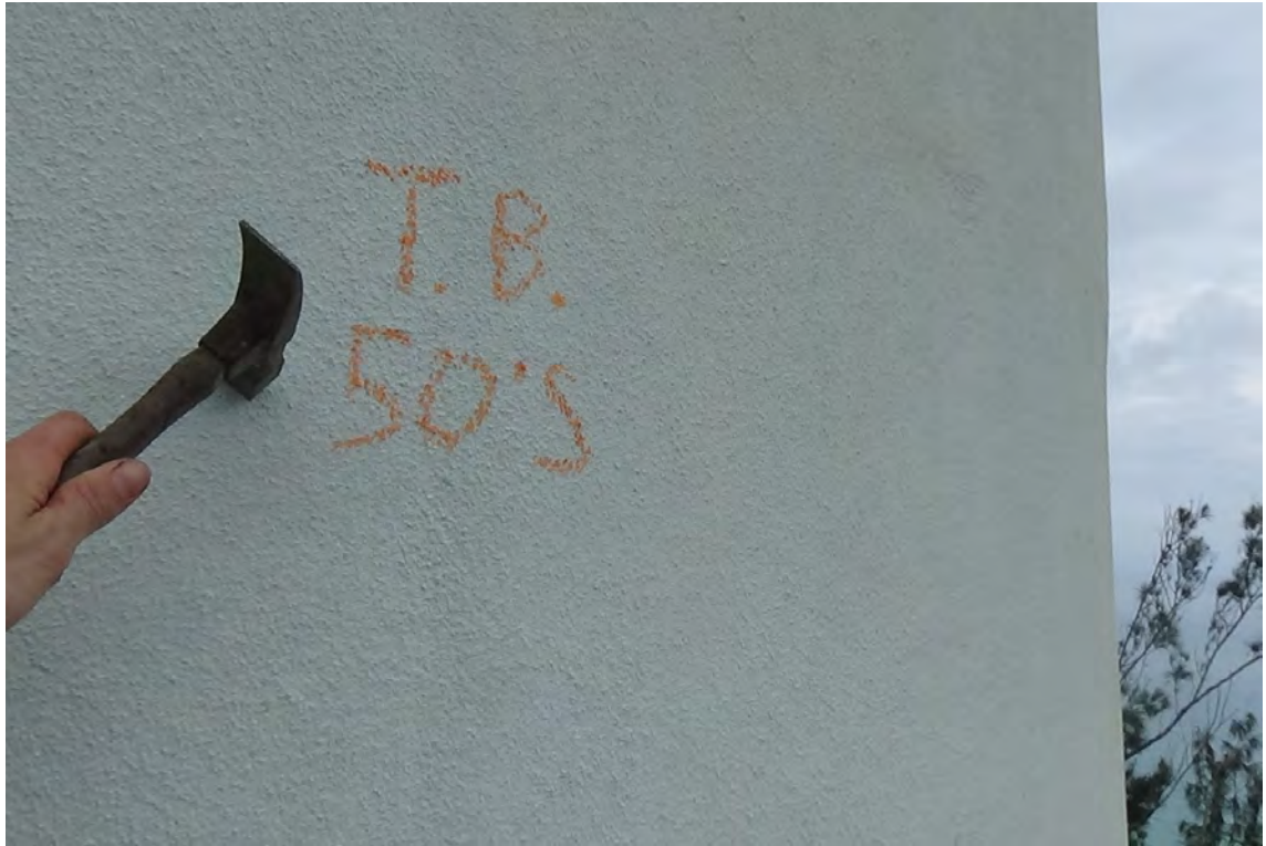
50' S—The concrete wall was hammer tested at various elevations to determine the composition and the hardness of the concrete. All the square footage which was observed and tested during the two exterior inspection drops, proved to be intact and solid.
