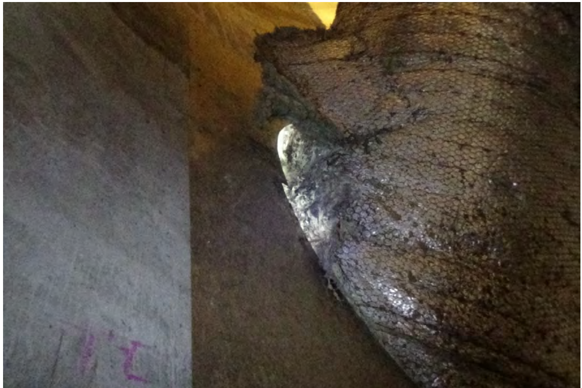
10' SE—Flue #1 breeching duct enters the concrete column on the south east side of the structure. A stainless steel plate is anchored to the concrete in order to minimize moisture penetration into the base. It appears as though the insulation has snagged on the cover plate at some point in time, tearing a small piece.
