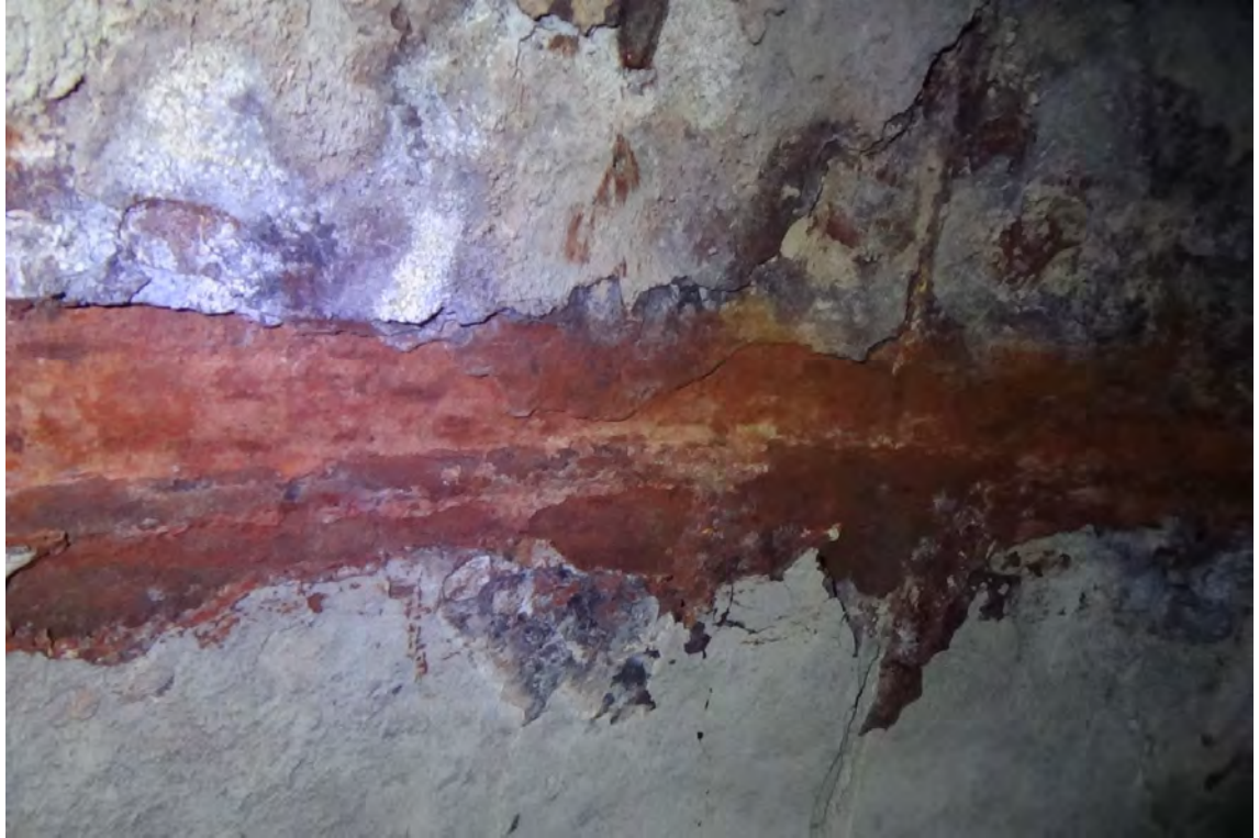
100' W/F1—Vertical and horizontal welds were cleaned and visually inspected at regular intervals. A heavy amount of scale was initially removed to view the weld. As was similar with other horizontal joints, the weld was found to be substantially rusted and pitted. Excess wear can best describe the condition of the weld.
