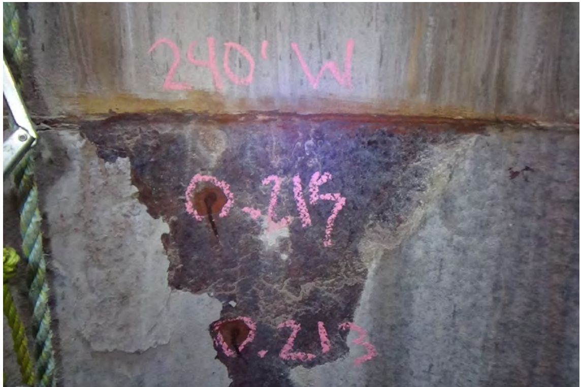
240' W/F1—Ultrasonic thickness measurements were taken at 1' intervals below the carbon to stainless transition. The measurements directly below the transition weld indicate approximately 15% steel thickness loss in the region.
