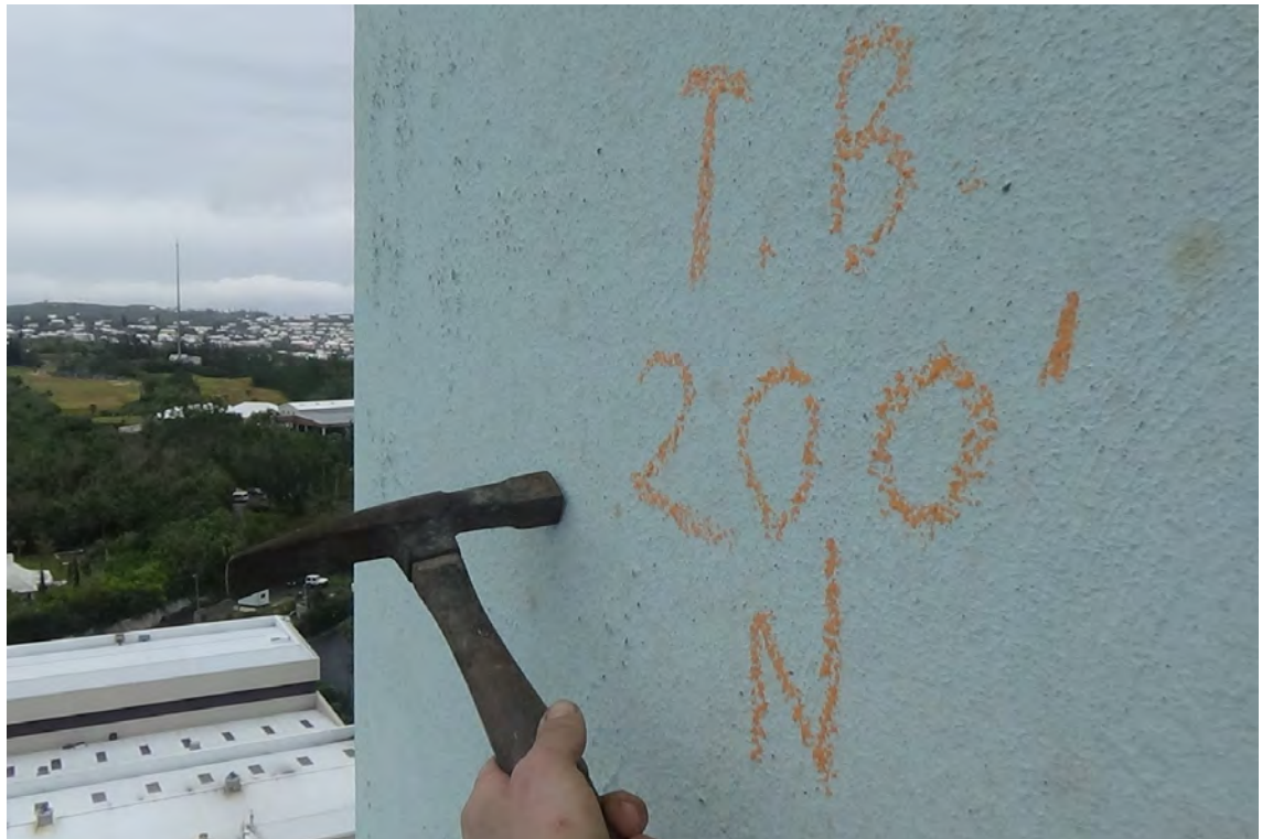
200' N—The protective coating below 200' is more consistent. Paint coverage was estimated to be 85% intact between the 150' to 200' elevations. The concrete was hammer tested throughout the height of the column and was discovered to be in sound condition.
