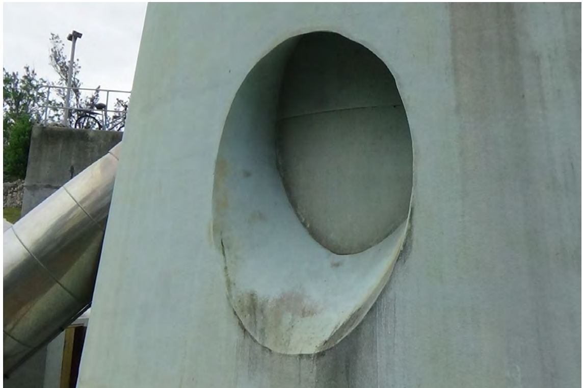
10' NE—Provisions have been made for a third flue to enter the column in this location. A cover plate has been anchored the interior wall to help keep out the elements and wildlife.
