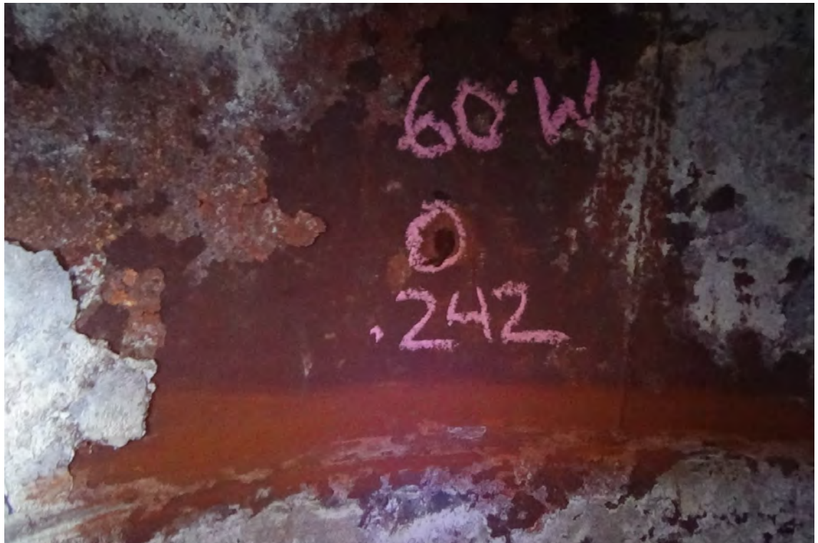
60' W/F1—Scale still needs to be removed to attain a UT measurement. Notice the outline of the scaling steel on the left side of the photo and the rusted surface beneath. The UT measurement taken is consistent with ¼" plate.
