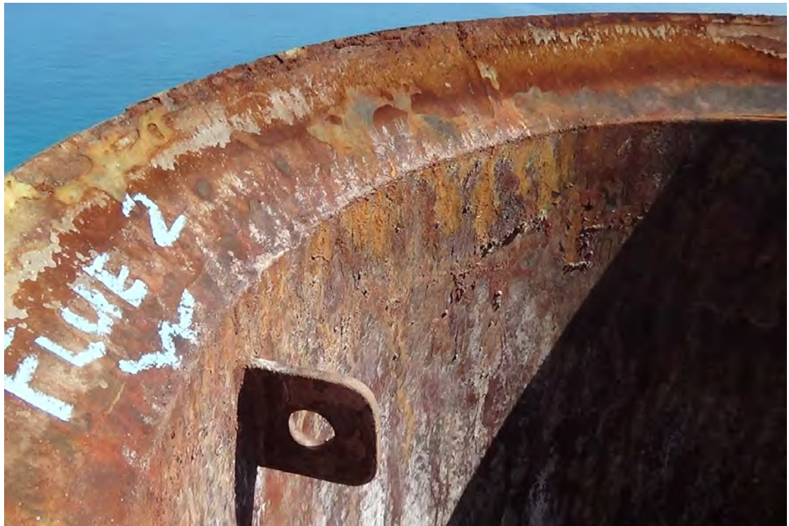
255' NE—A crack approximately 3' long was observed in the weld connecting the cap to the liner wall on flue #2. The corrosion at the top of flue #2 appears to be more profound than that of flue #1.
