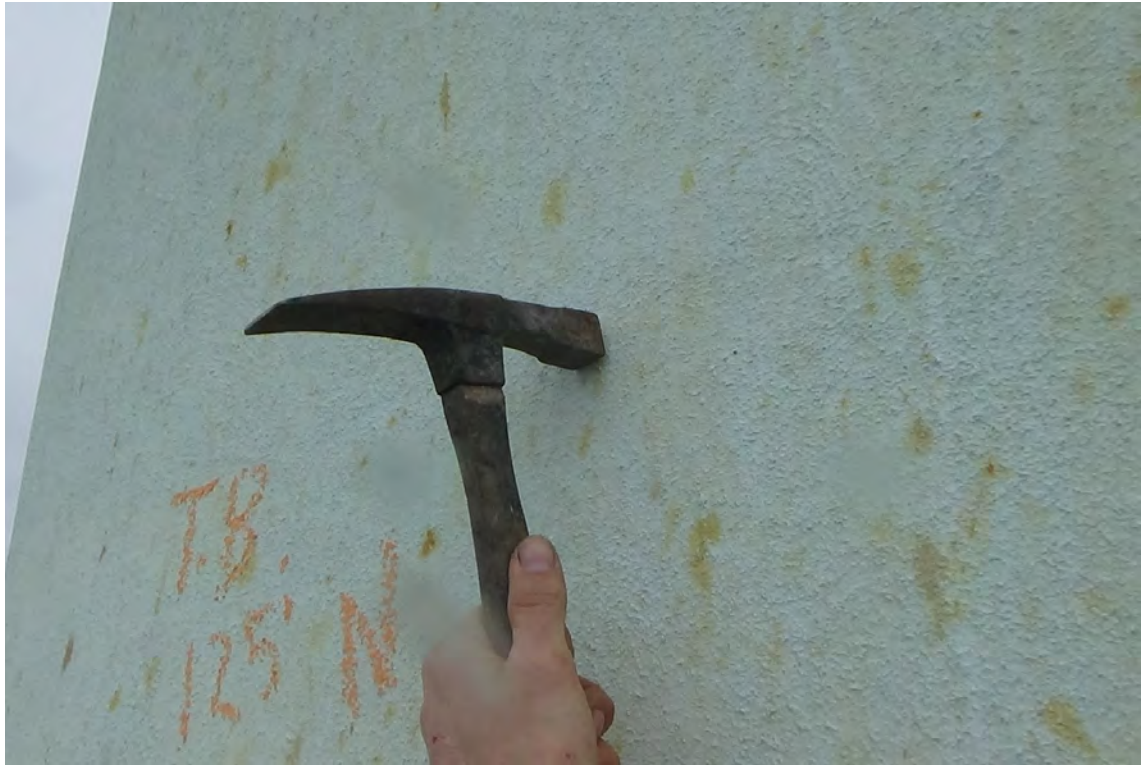
125' N—The exterior of the concrete column was found to be in excellent condition throughout the height of the structure. No cracks or evidence of spalling were observed during the north inspection drop.
