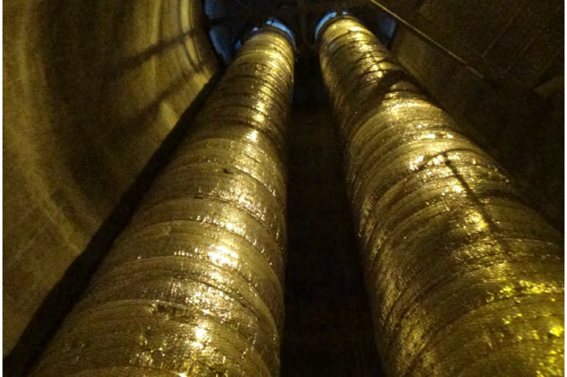
100' E—View looking up at the flues indicates no damage or deterioration to the insulation and wire mesh encapsulating the two flues.
