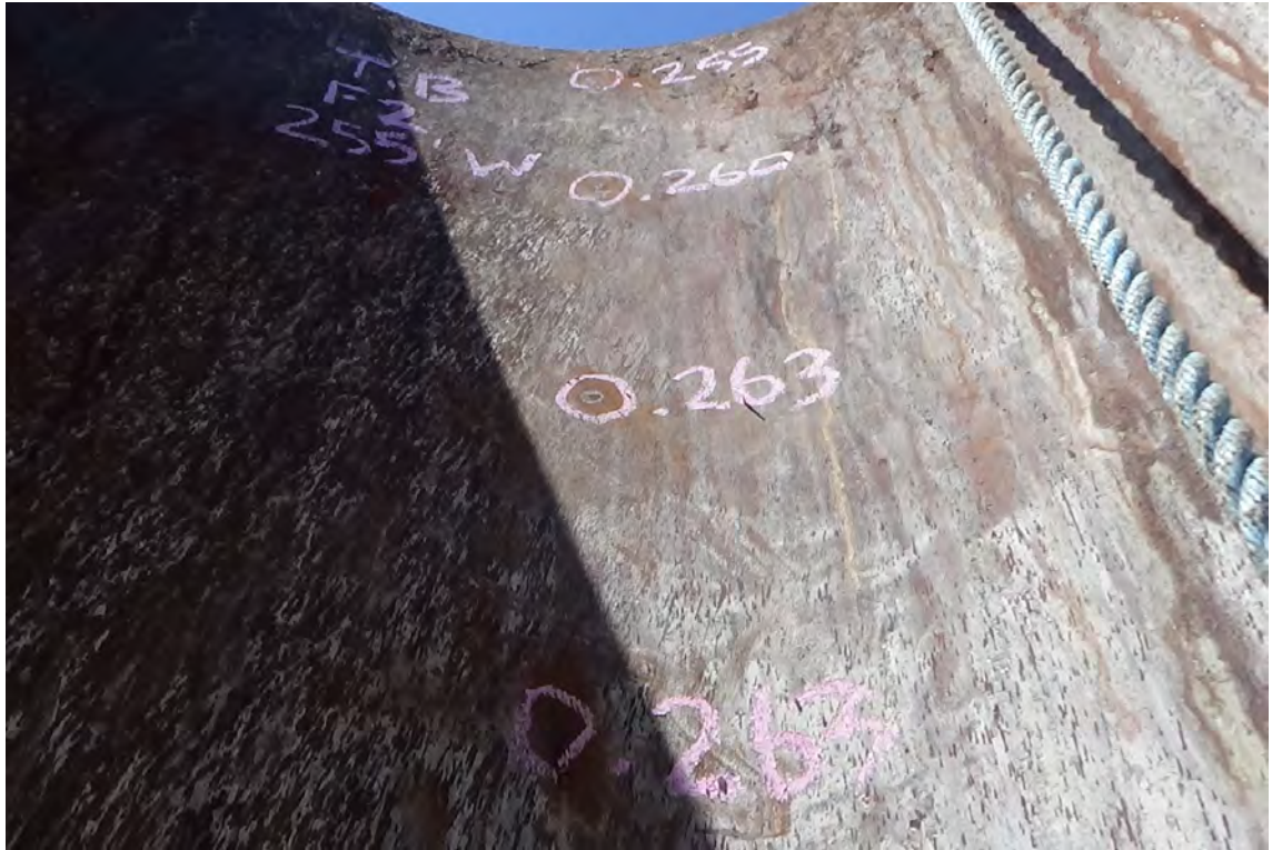
255' W/F2—UT readings were taken at 1' intervals throughout the top 10' of the liner. Measurements were then taken at 10' intervals for the remainder of the flue. All measurements taken within the stainless steel portion closely correspond to ¼" thick plate.
