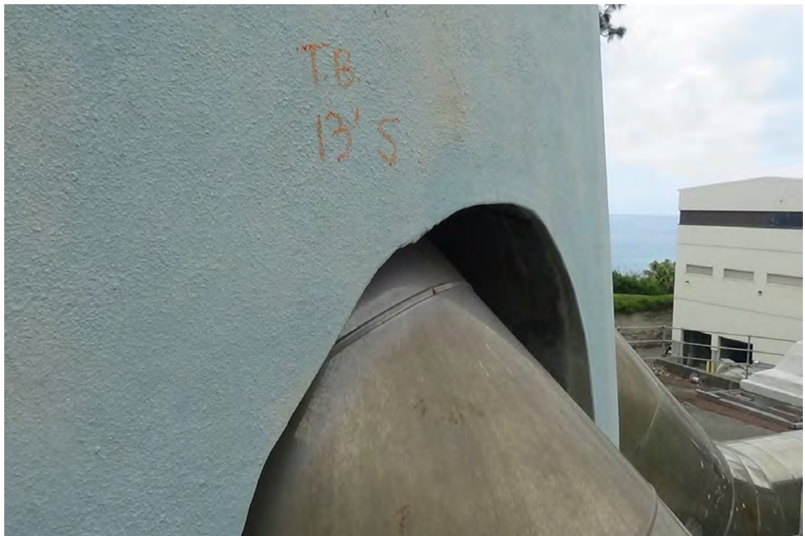
13' SE—Flue #1 enters the concrete column. No deficiencies were noticed around the opening or on the duct cladding.
