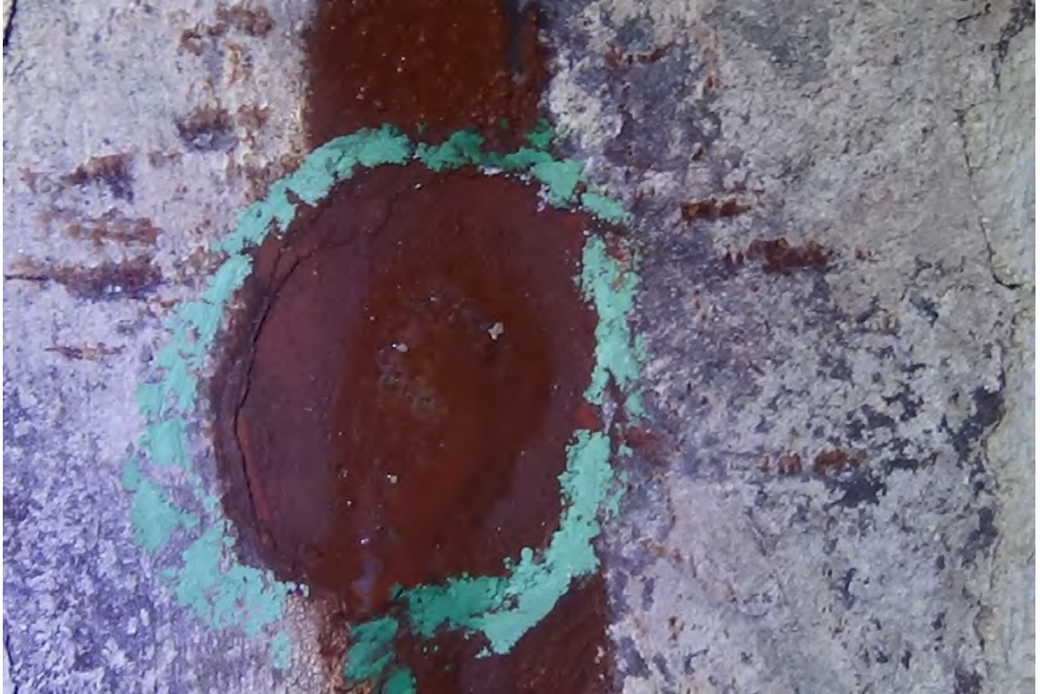
190' W/F2—Multiple layers of scale was removed before UT readings could be taken. Notice the pitting located within the clean steel.
