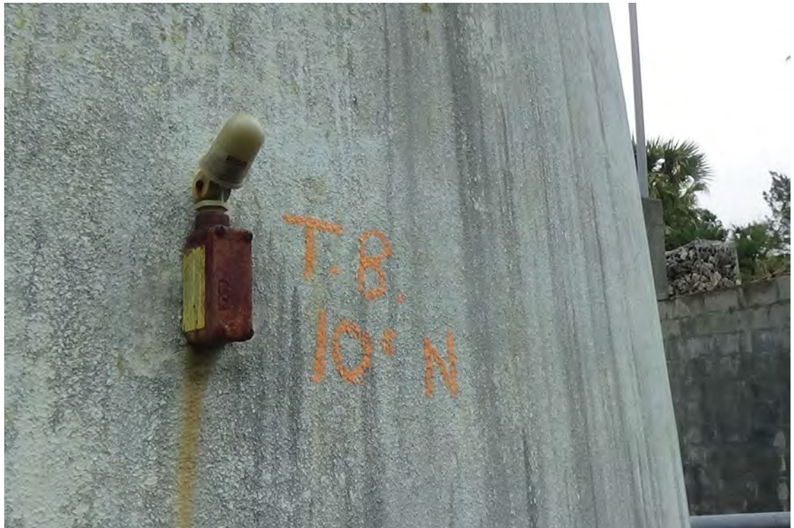
10' N—A small electrical junction box appears as though it once housed an exterior light or intended to. The junction box is moderately rusted and pitted, the pivot head was found to be damaged.
