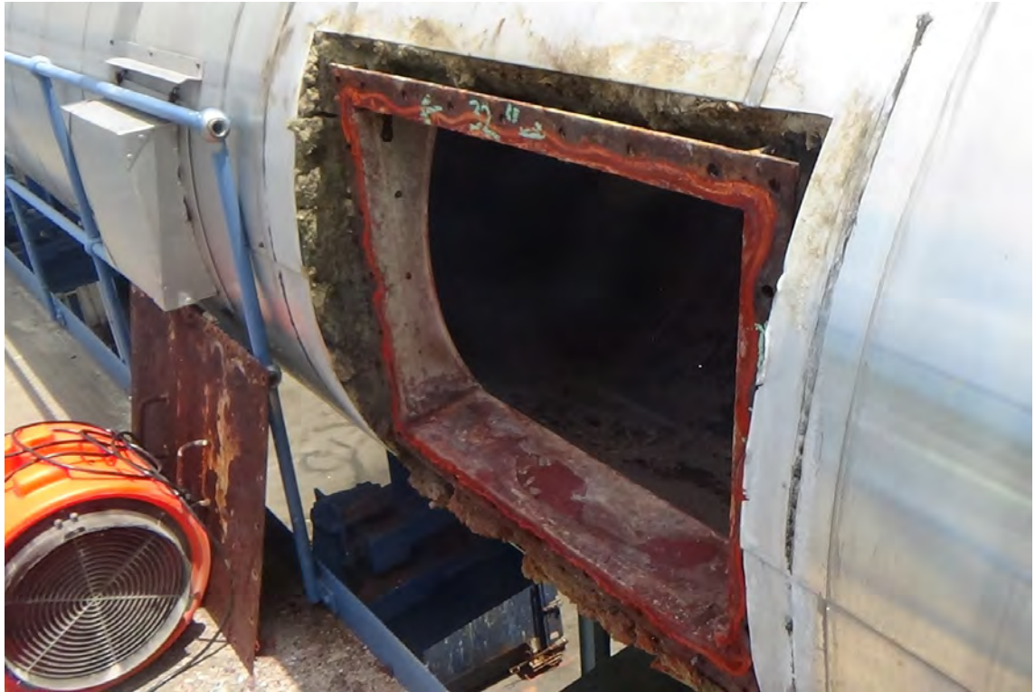
4' N/F2—The access door to flue #2 is located in the horizontal breeching duct approximately 30' from the base of the chimney. The opening measures 32" by 25". All the ½" bolts securing the access door were extremely corroded and were cut with a grinder/torch in order to remove the door.
