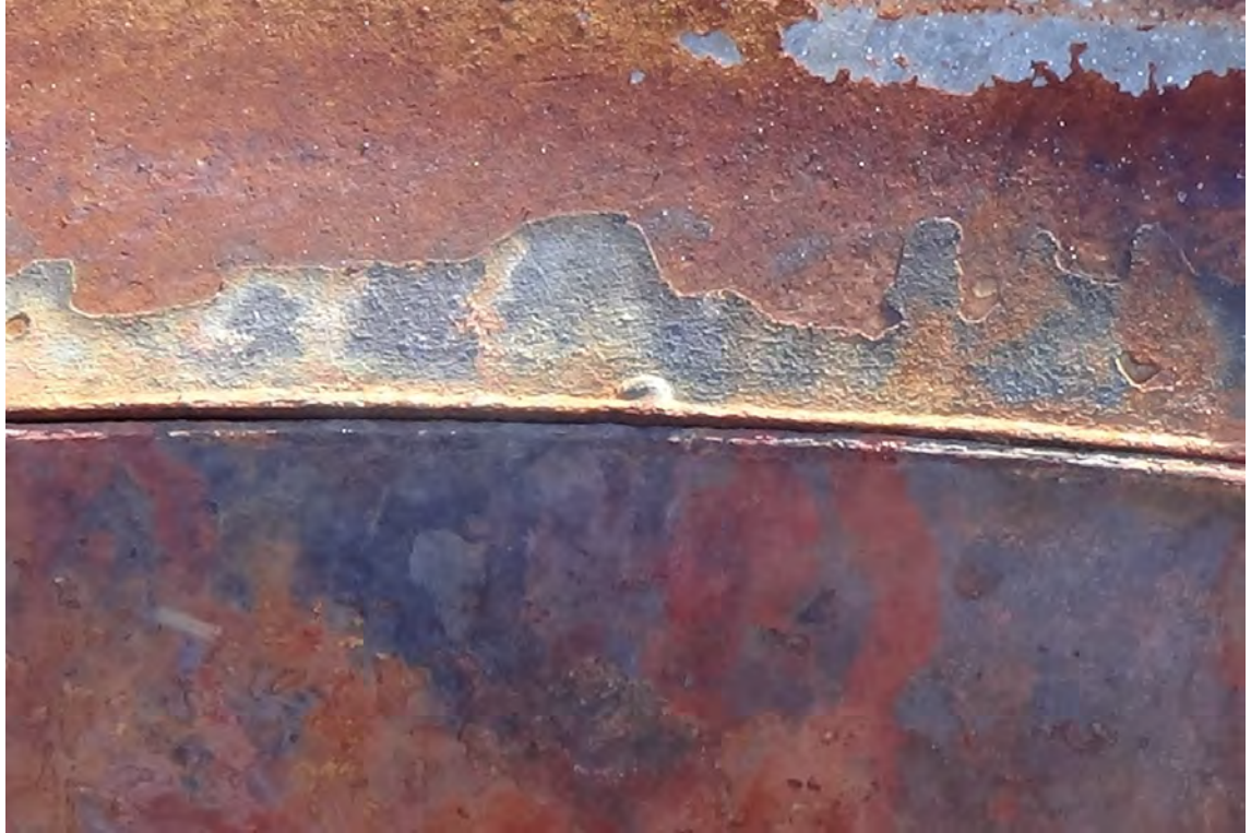
255' E—Close up photos of the cracked weld which attaches the rain cap to the interior flue wall. This particular crack continues for approximately 3'-0".
