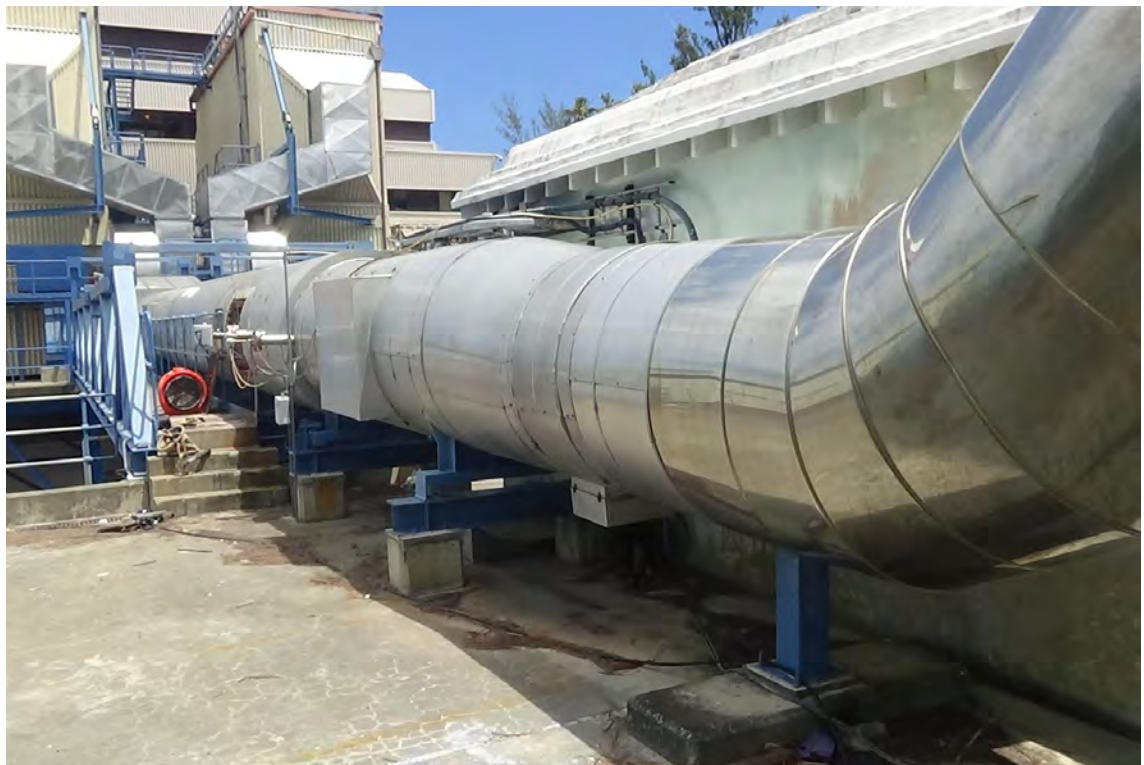
0' E/F2—The flue access door is approximately 30' away from the base of the chimney. The access door is the opening near the stairs to the bridge.
