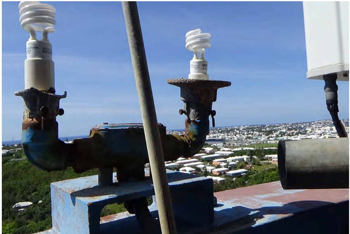
250' S—The red globe on the right side of the AOL was found to be unsecured, the casing on the light on the right was discovered to be cracked 360°. Both globes were removed to eliminate a falling object hazard. They were later replaced and secured with electrical tape as a temporary fix.
