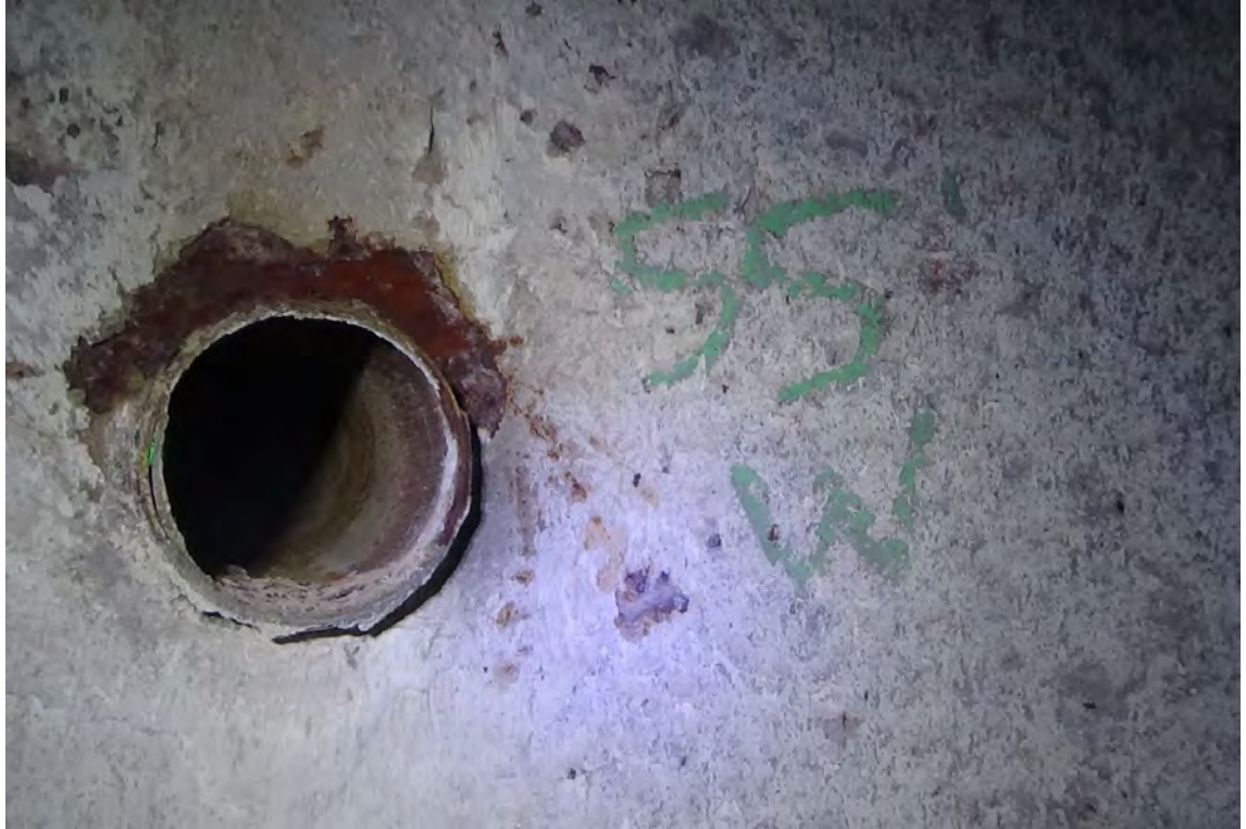
55' W/F2—Opacity meter test port displays minimal process build-up inside the port hole. Test ports appear to be solely welded from the exterior.
