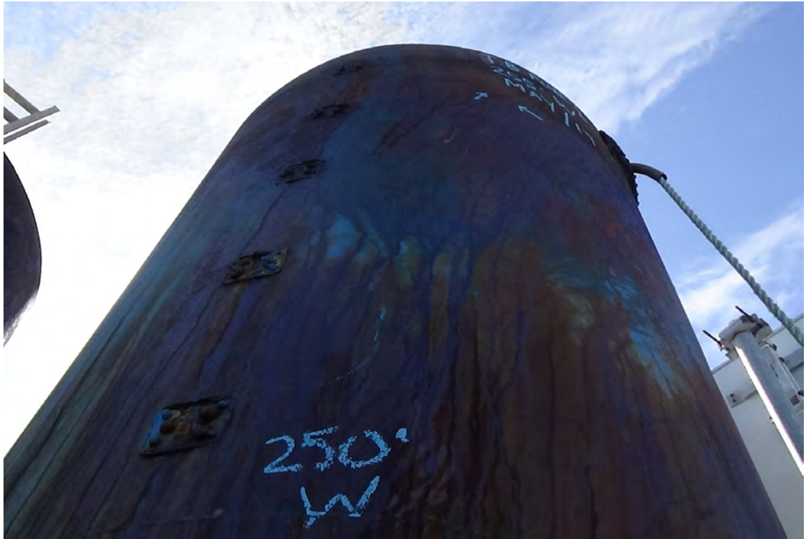
250' W—The exterior cladding of flue #1 was painted blue in the past. A minimal amount of original paint is still visible. The top 5' of the cladding displays a moderate amount of corrosion. Pock marks within the cladding are near penetrating through to the insulation underneath. Corrosion holes are visible near the top.
