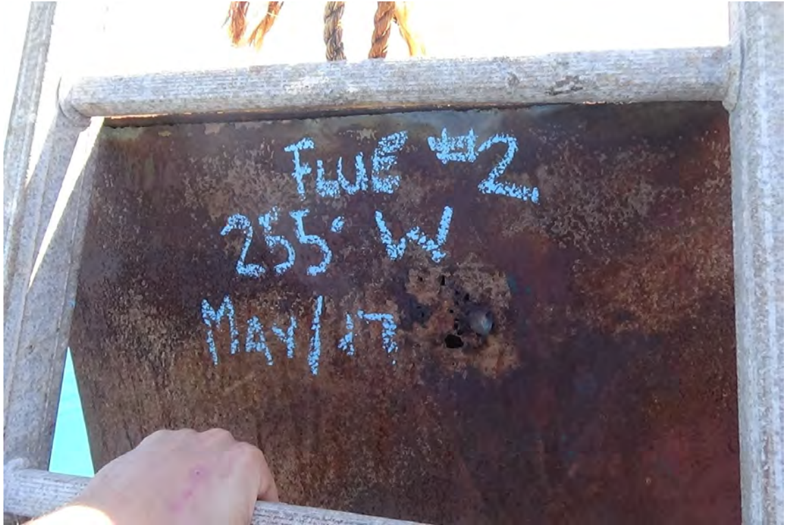
255' W—The top 5' of the stainless steel cladding on flue #2 is severely corroded. Approximately 300° of weld connecting the rain cap to the cladding was found to be cracked causing a large misalignment between the two components.
