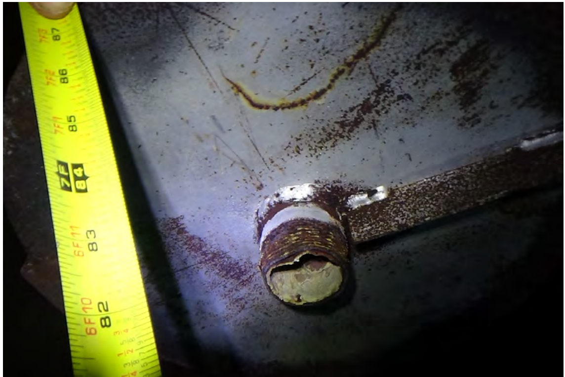
7' E/F1—The hopper portion of the false floor was measured to be 7' from the base of the liner. The nozzle on the hopper is open and appears to be corroded. A look up into the nozzle displays the scale build-up visible from within the flue.
