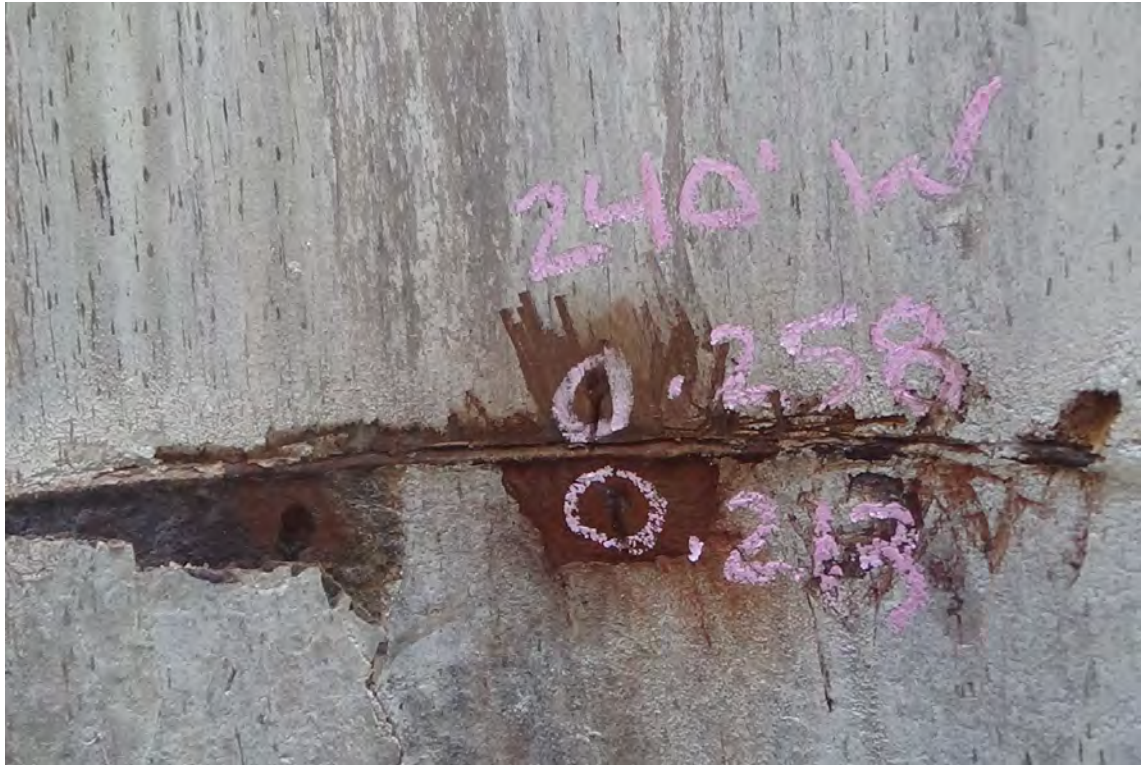
240' W/F2—UT readings taken above and below the transition weld illustrates the moderate steel thickness loss within the carbon steel section of the liner. The reading taken (.213) represents an approximate 15% loss in plate thickness at this elevation.
