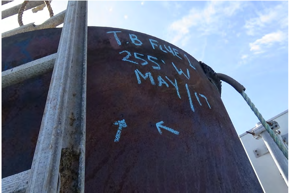
255' W—The top of flue #1 displays a moderate amount of pitting and corrosion within the top 5' of the stainless steel cladding. The blue arrows point to corrosion holes in the cladding.
