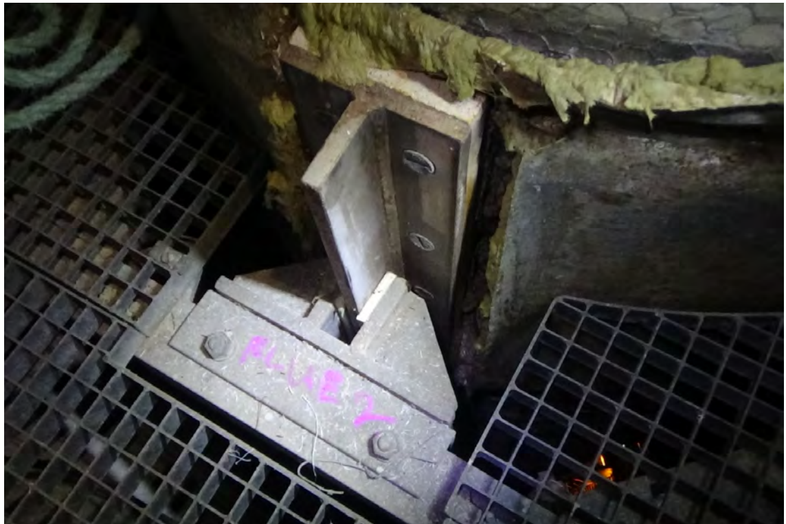
200' E—Each liner is furnished with four horizontal stabilizers located 90° from one another. These stabilizers consist of a system to keep the liners centered and allows for the liners to expand and contract during thermal expansion. All stabilizers were found to be intact, with all components in sound condition.
