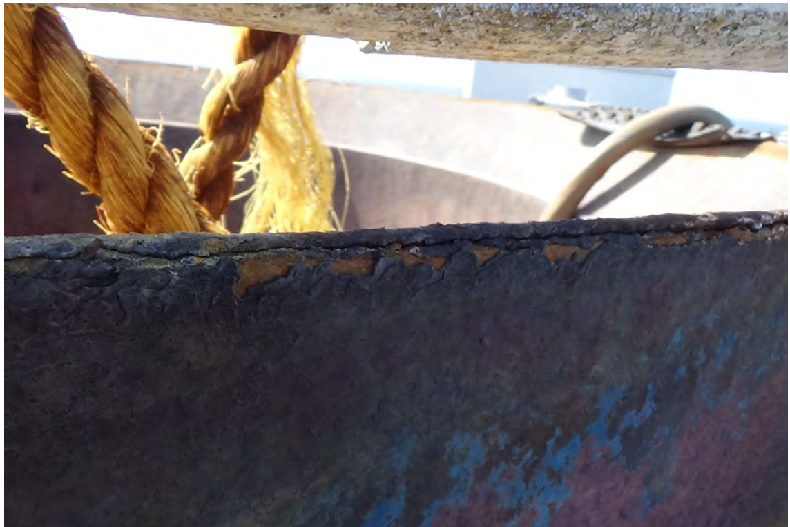
250' NW—Close-up of the cracked weld mentioned in the photo above. The crack continues for approximately 5'-0". The corrosion below the crack appears to be deteriorated paint.
