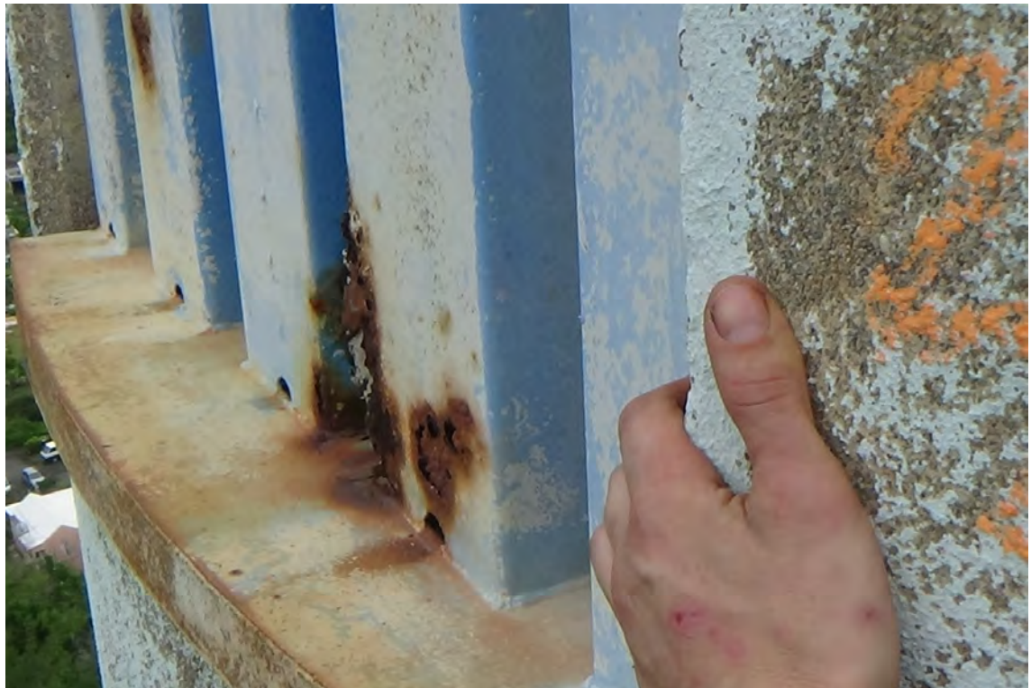
242' S—The paint on the vent cover is weathered. The paint on the vents displays approximately 15% coverage. In areas where the primer coat has deteriorated rust, scaling and corrosion holes are visible.
