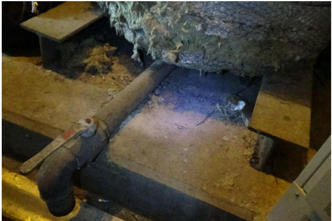
1' N—A steel drain pipe exits the base of flue #1. The drain pipe has a valve in order to remove standing water from the base of the liner. This drain works in conjunction with the hopper drain for the base of the flue. Both drain pipes appeared to be clogged at the time of the inspection.
