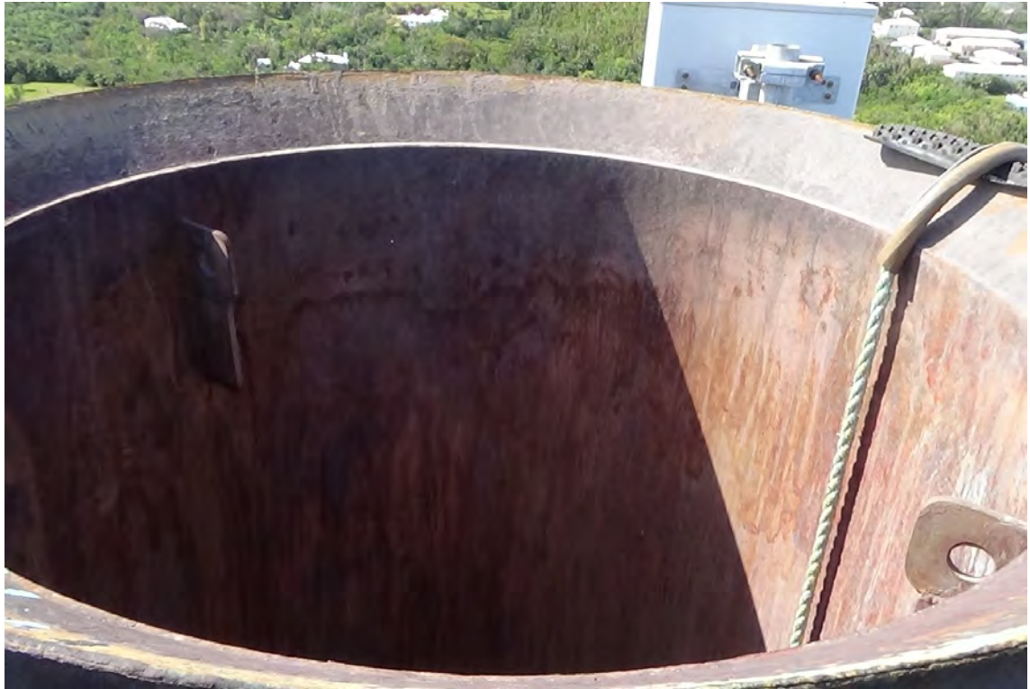
250' S—View looking across to the top of flue #1. A crack in the weld connecting the rain cap to the cladding can be seen in the very bottom right hand corner of the photo.
