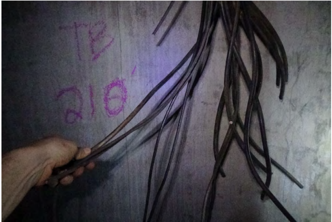
210' W—The wiring for the obsolete satellite transmitters has been severed at this elevation. The loose wires have been left hanging in the annular space.
