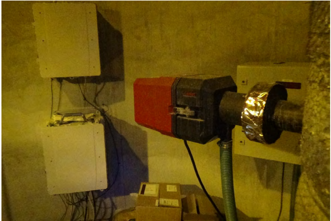
50' N—Photo of the new opacity meters which were installed during the same time as the 2017 inspections were being performed.
