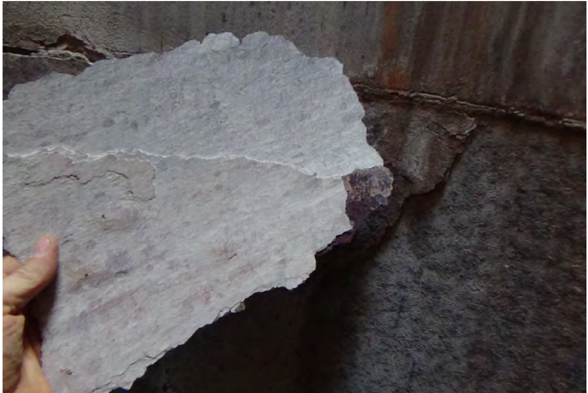
240' W/F1—Heavy scaling is visible to the carbon steel wall beneath the carbon to stainless steel transition. The scale was easily removed from the liner wall as is evidenced from the large piece being displayed by the inspector. The heaviest amount of scale was found near the top of the carbon steel portion of the flue.
