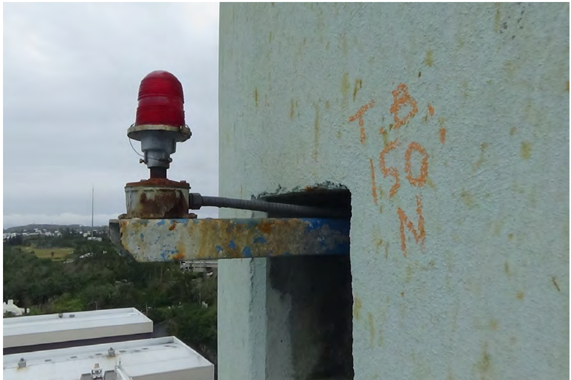
150' N—Aircraft obstruction light is in satisfactory condition. The bottom casing is significantly rusted and showing signs of corrosion. The blue paint covering the mounting channel is approximately 25% in tact. The light appears to be off during the daytime hours.
