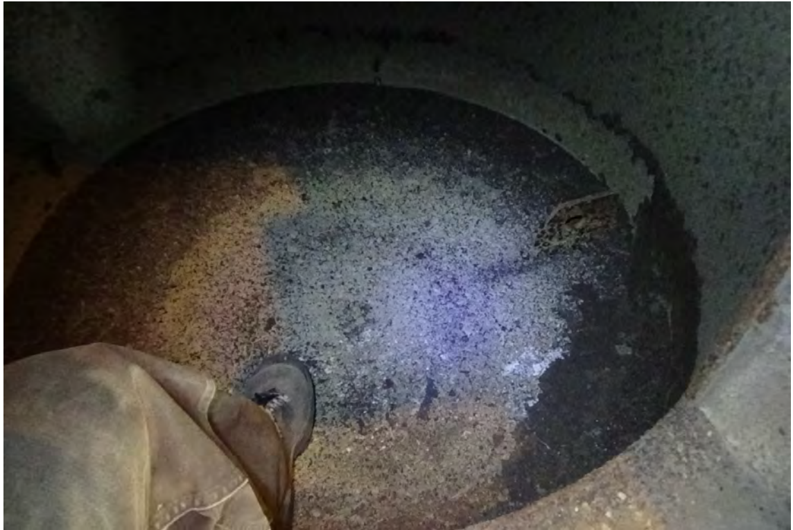
0' /F1—The build-up in the bottom of flue #1, under the false floor is extremely hard. The drain in the middle of the floor is plugged with a concrete like substance.
