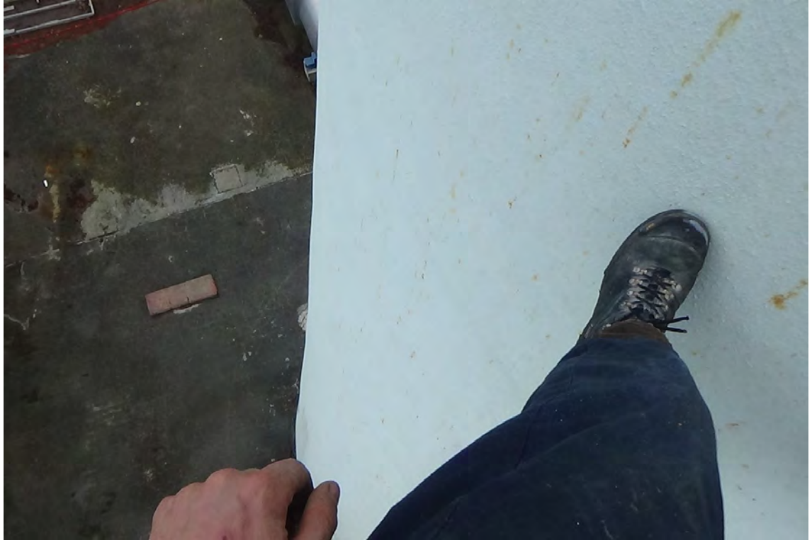
50' N—View looking down towards the base of the chimney displays minimal amount of paint staining at lower elevations. The concrete wall tapers outwards below this elevation
