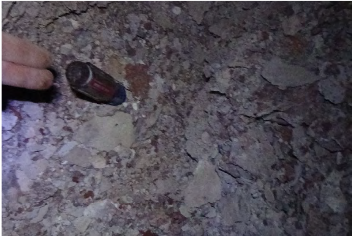
10'/F1—A substantial amount of scale and debris build-up was found in the base of flue #1. A depth measurement of the build-up was attempted. The measurement was found to be over 16" of build-up. The false floor wasn't reached.
