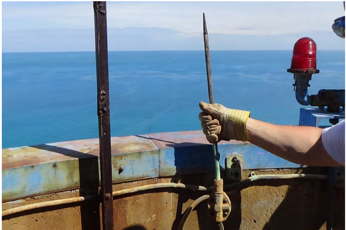
250' N—A stray lightning point was found to be tied into the LPS on the north side. The point is not mounted and was discovered to be tucked in behind the angle iron seen on the left side of the photo.
