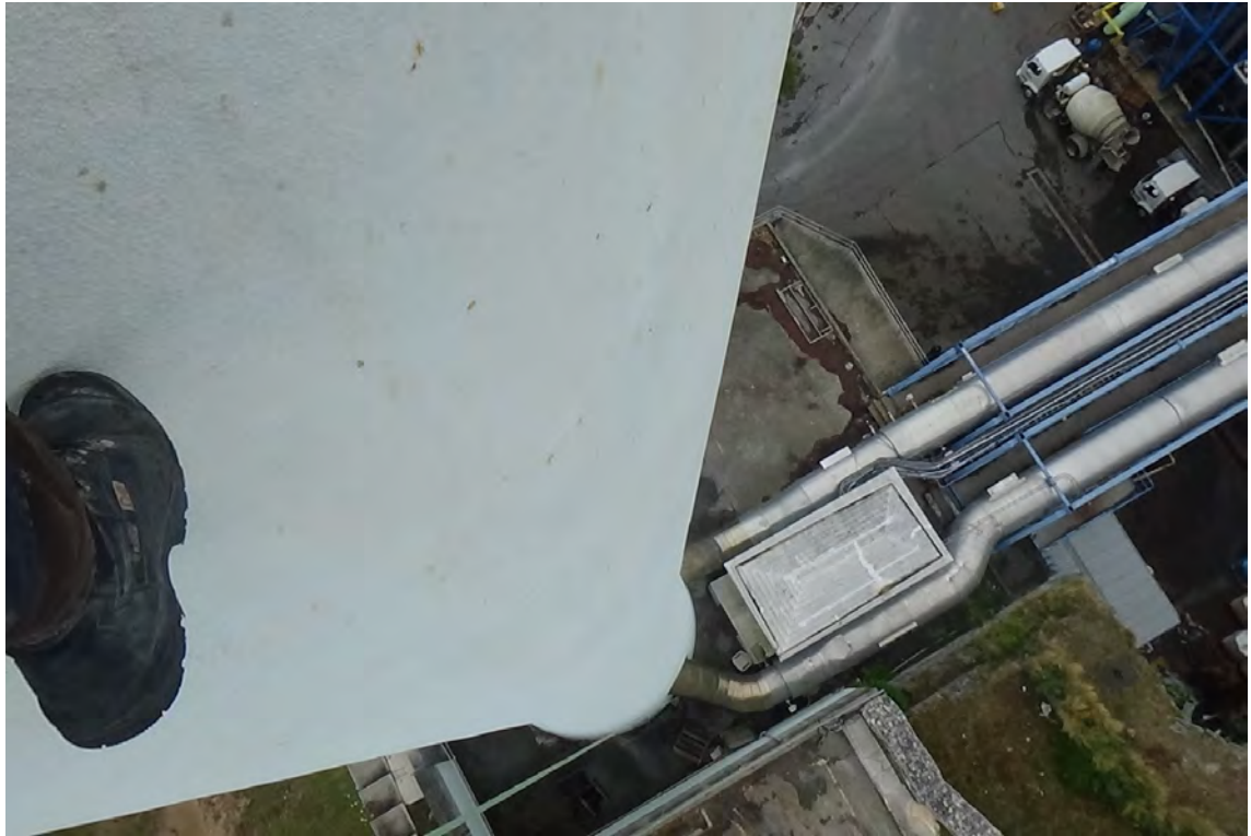
125' S—View looking down the wall shows significantly less staining to the paint than at higher elevations. Breeching ducts enter the concrete column on the east and south east sides of the structure.
