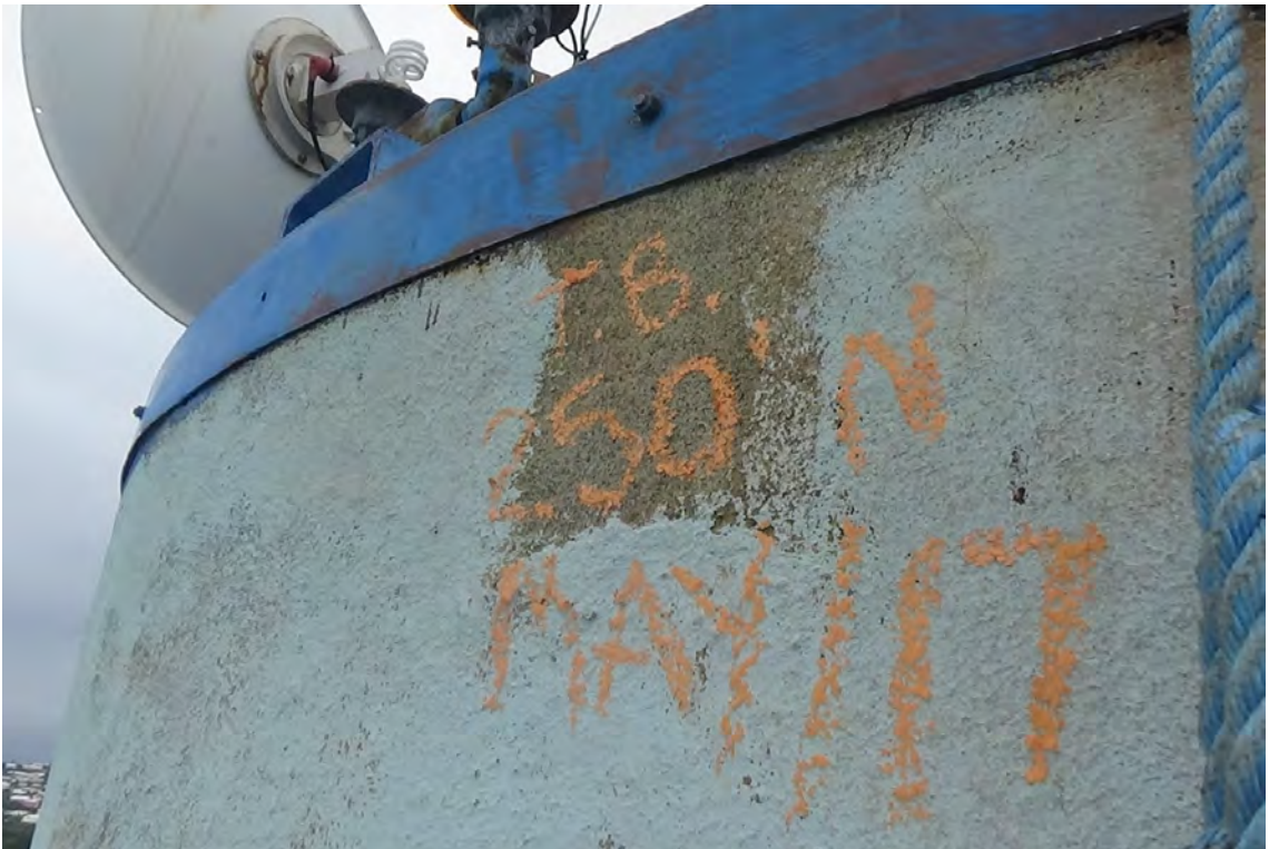
250' N—Area of bare concrete is visible where rigging would have been placed during original painting of column. The protective coating is badly worn throughout the top 50' of the chimney.
