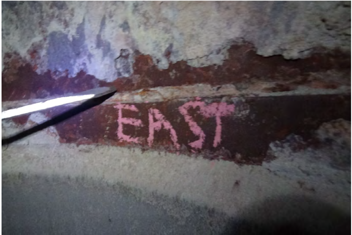
30' E/F1—The horizontal joints above and below the slider sections appear to be welded from the exterior of the flue. The joint has either been sealed with a high temperature cement or has accumulated process material over the years. The material filling the joint was found to be hard and mostly intact.
