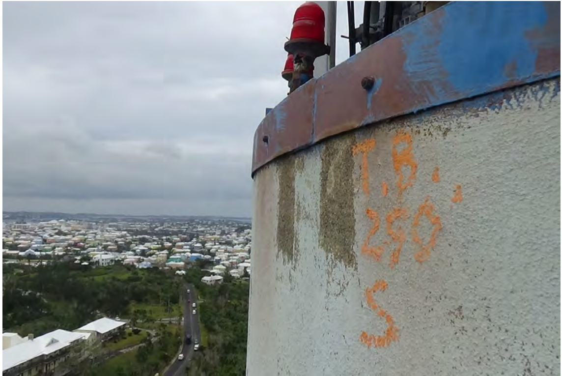
250' S—Two small areas of bare concrete are noticeable below the rain cap. Paint on the cap is badly worn, red primer is visible beneath blue top coat. Aircraft obstruction light casing appears cracked and severely deteriorated.
