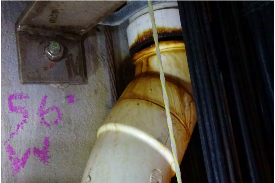
156' W—A break in the drain pipe was visible at this elevation. It appears as though the PVC pipe has cracked at a connection point leaving a \frac{3}{8} " gap, 360° around the pipe.
