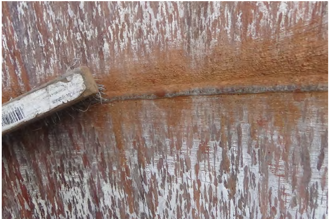
250' W/F2—The horizontal welds within the stainless steel portion of the liner were found to be consistent with a smooth profile. No cracking or other deformities were noticed. There does appear to be a mild amount of pitting to the stainless above and below the weld.
