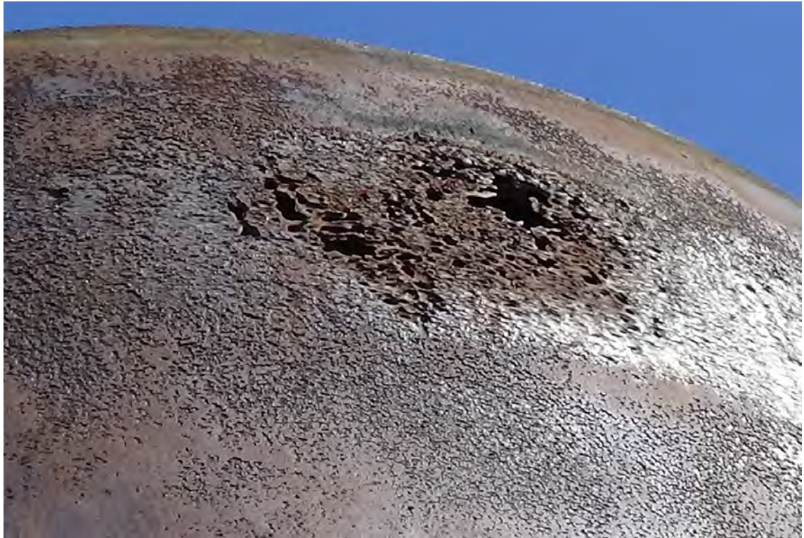
255' S—Large area of corroded cladding on the south side of flue #2. The pitting of the stainless steel is very noticeable in this location.
