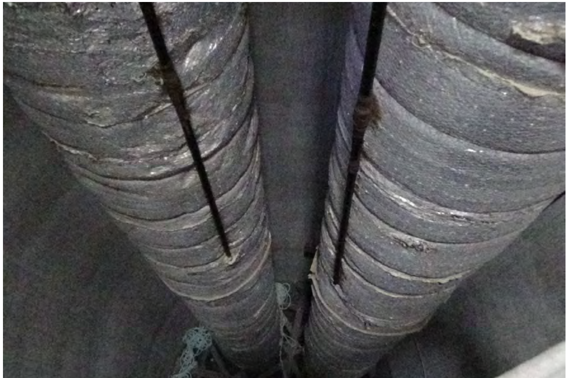
230' E—View looking down the flue ducts towards the connection between the flue suspension bars and the liners. The insulation and wire mesh is generally intact throughout the top 50'. Small tears are noticeable in localized areas.
