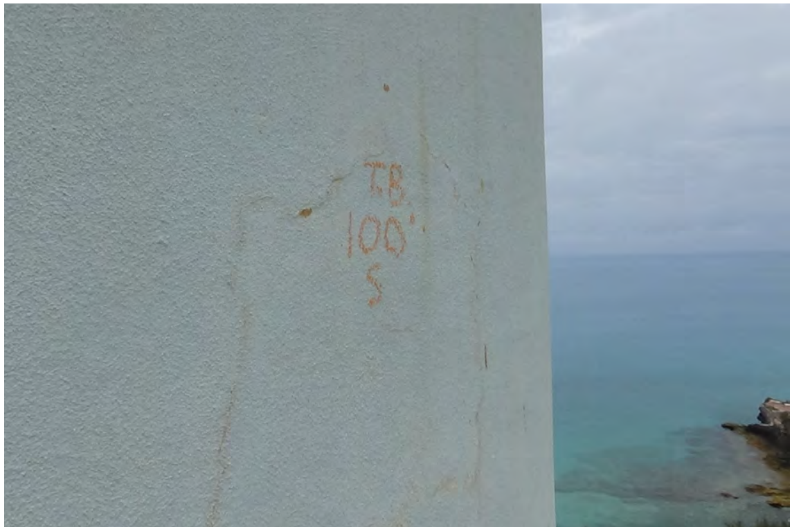
100' S—A series of hairline cracks are visible within the concrete. These minute cracks form a circle approximately 2'-0" by 1'-6" in size. The concrete inside and around the defect was tested with a hammer and found to be solid.
