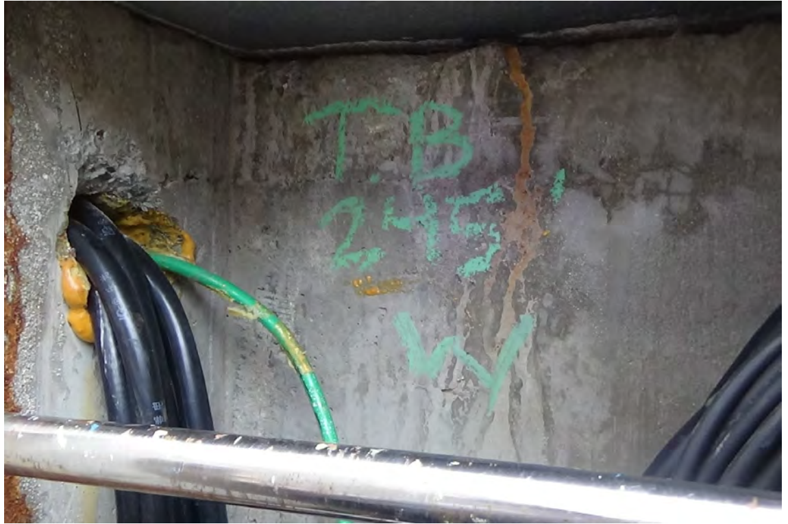
245' W—Expandable foam was used to seal the holes where the electrical and satellite cables exit the concrete column. Much of the foam appears to have deteriorated leaving a slight void behind.
