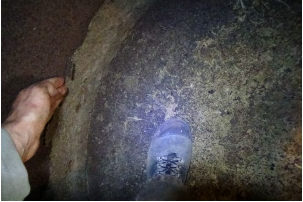
0' S/F2—A ring of scale approximately 6" wide is visible in the base of liner #2. This deficiency suggests that standing water was present in the base in the past.
