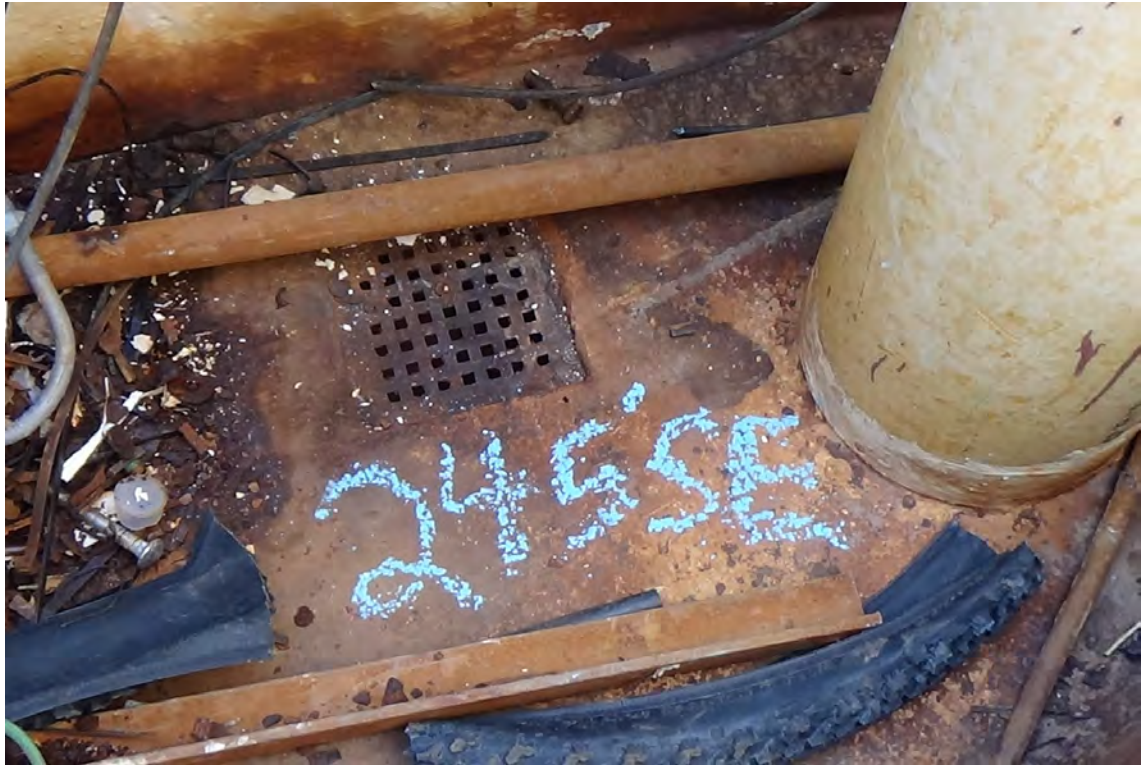
245' SE—The drain cover on the south east side is free of obstructions. The cover plate is level with the concrete floor and appears to be functioning properly. Notice the amount of trash and debris that has accumulated on the roof over the years.
