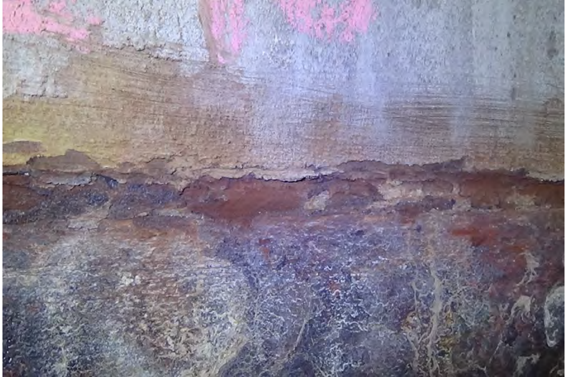
240' W/F1—Heavy scale needed to be removed from the transition weld in order to perform a visual inspection. The weld is extremely rusted and pitted, a significant amount of undercut is visible within the stainless steel portion of the liner. No cracks or separation were visible within the weld.
