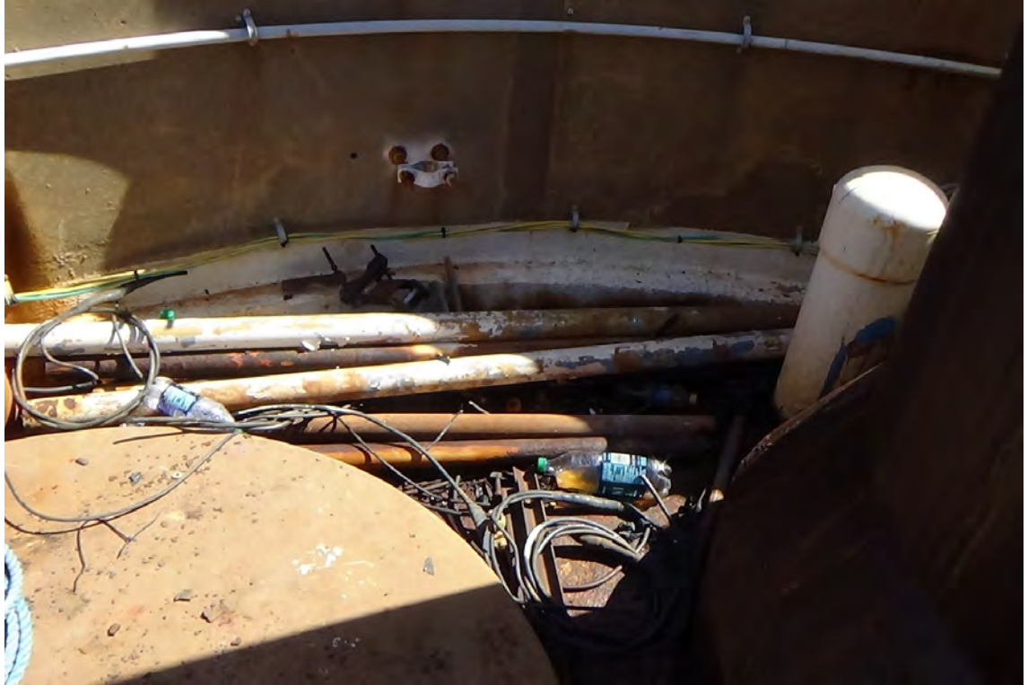
245' N—Trash and scrap material has compiled on the roof deck giving an air of untidiness and creating tripping hazards.
