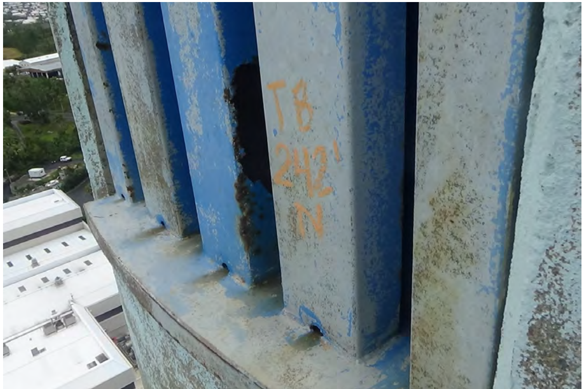
242' N—The blue paint protecting the steel vent cover appears severely weathered. Paint coverage on the steel cover was estimated to be 50% in tact. Areas of significant rust and pitting are visible on the steel channels.
