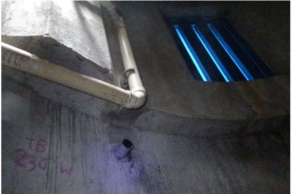
230' W—The drain pipe below the roof elevation is fully intact and properly secured. Notice the interior wall thickness increase of 7\frac{7}{8} ". This wall increase is necessary to carry the weight of the roof slab, carrier beam and flues.
