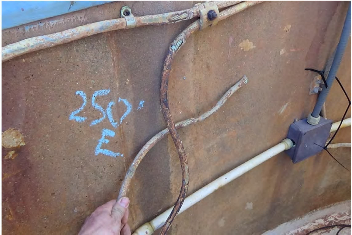
250' E—A disconnected ground cable was found to be tucked behind the electrical conduit. The cable is believed to have serviced flue #2. There was not a ground connection on flue #2 found during the inspection. Notice the wear to the lead casing on the ground and circuit cable.
