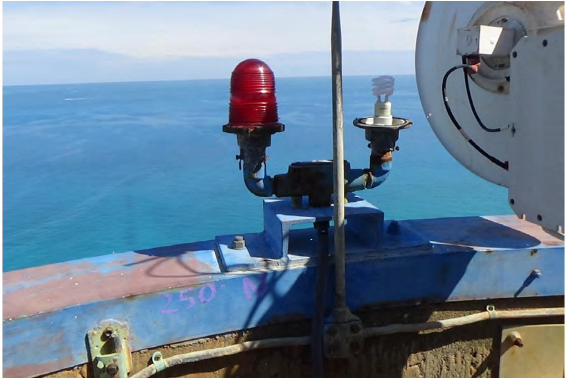
250' N— One red globe on the north side light was found to be missing. Red pieces of glass were discovered on the concrete roof slab, suggesting that the globe fell inwards.
