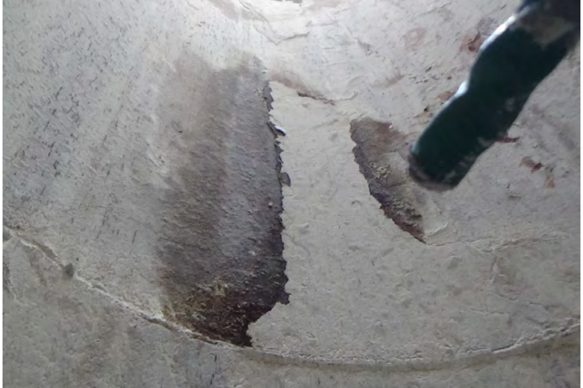
230' S/F2—Loose scale was removed from previous picture. Beneath the loose scale the carbon steel wall appears extremely rusted with multiple layers of scale.
