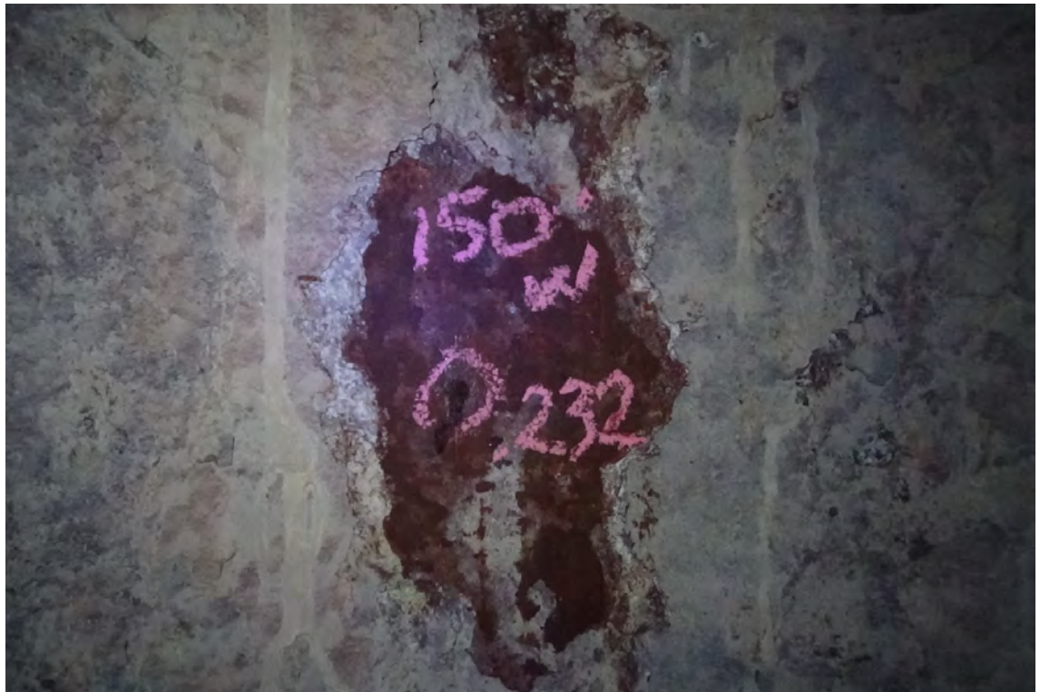
150' W/F1—Another area of heavy scale was removed in order to record a proper UT measurement. Please refer to Section 3 in the inspection report for a chart referring to elevations, thickness readings taken and original design specifics.
