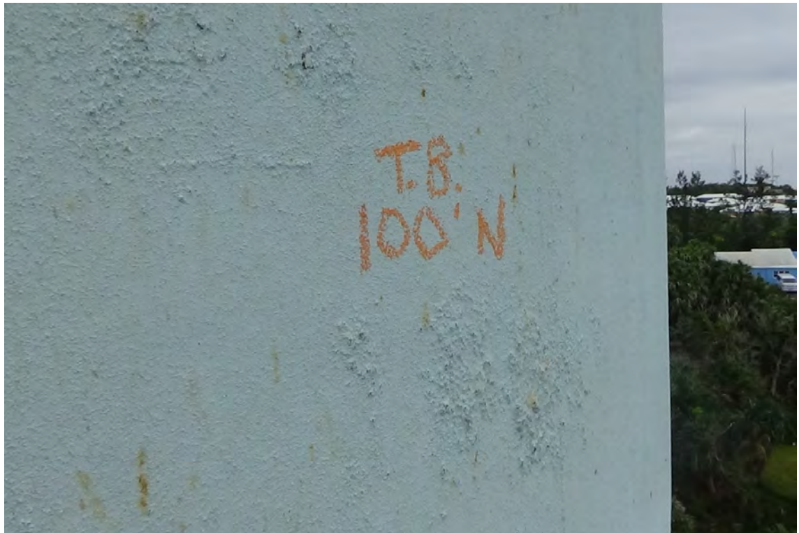
100' N—Areas of rough concrete were observed in this localized area. This minor deficiency can be attributed to concrete sticking to the forms during the original slipforming of the column. These areas were tested with a hammer for hardness and were found to be solid.
