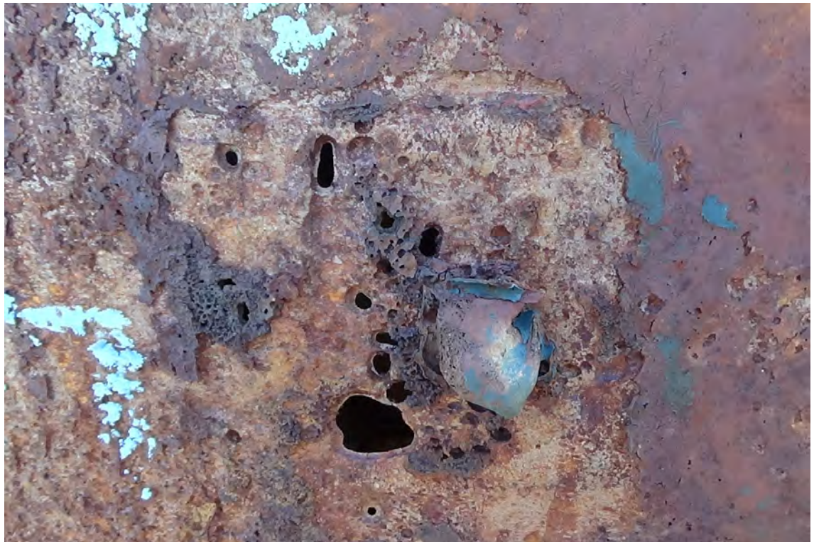
255' W—Small corrosion holes are visible in the stainless steel cladding throughout the top of flue #2. The insulation between the cladding and the liner wall is partially exposed.
