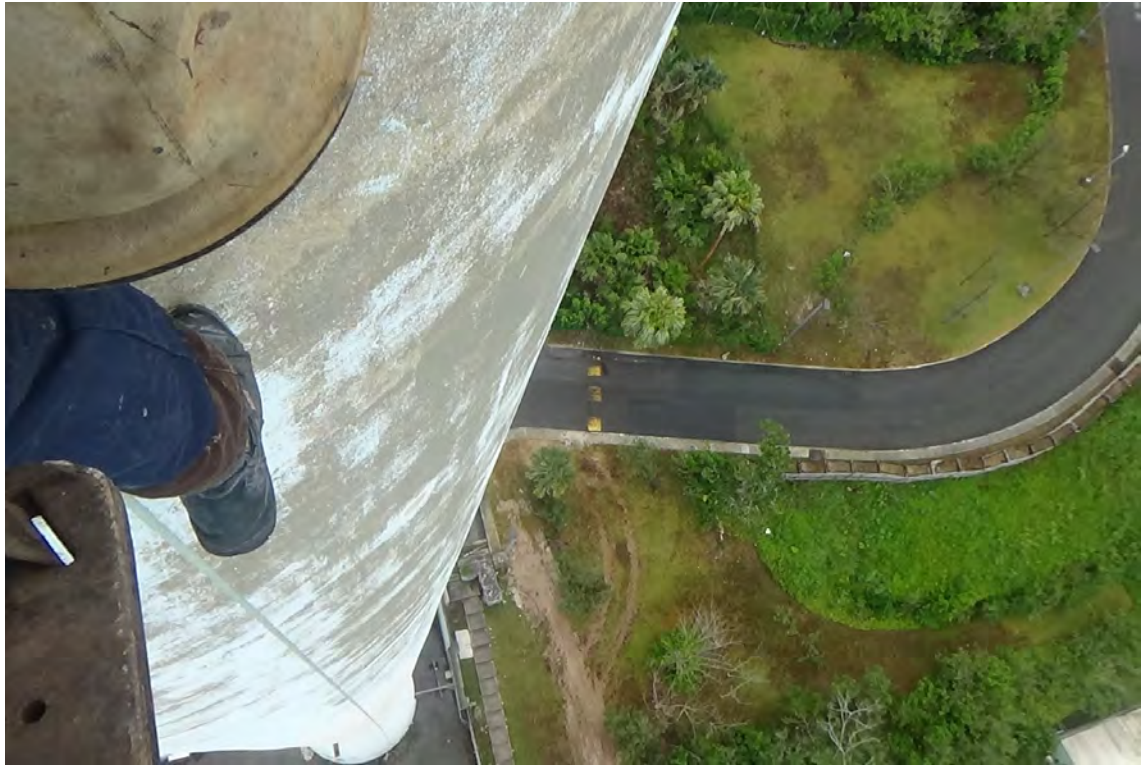
250' N—View looking down the exterior of the concrete column displays significant paint deterioration. Paint coverage within the top 50' was estimated to be 30% in tact.
