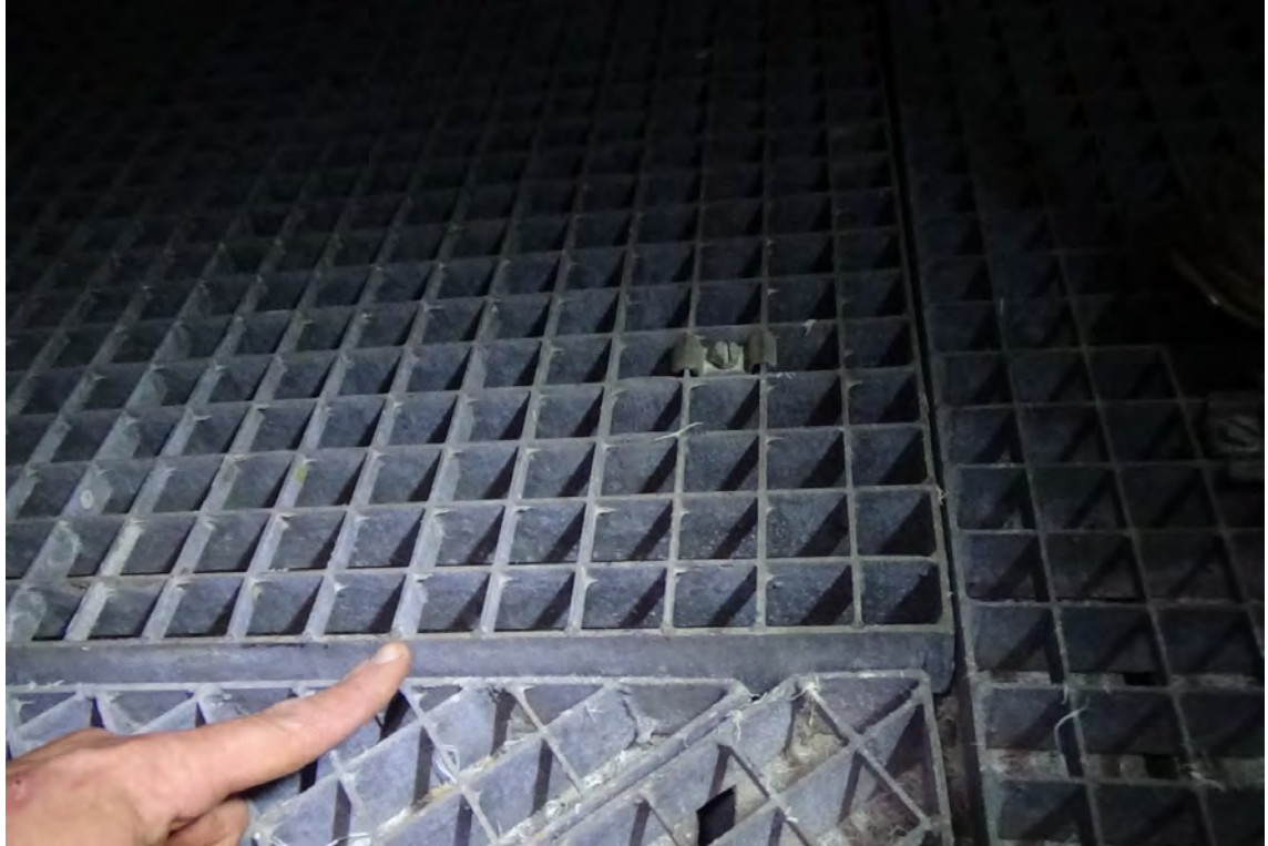
200' N—The grating which is located within the bay allotted for a third flue, appears loose and misaligned with the rest of the grating on the platform. It is believed that this grating is removed from time to time to hoist material to the upper elevations.
