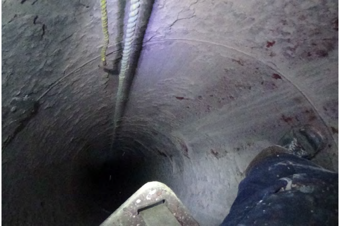
190' W/F1—View looking down the liner displays a consistent amount of scale throughout the height of the liner. The scale is easily removed from the wall in large sheets.
