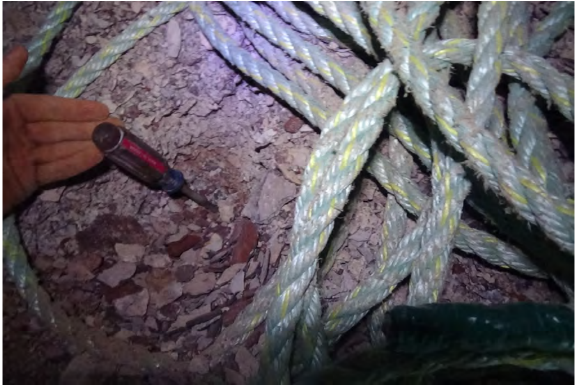
10'/F2—A substantial amount of scale and debris build-up was found in the base of flue #2. A depth measurement of the build-up was attempted. The measurement was found to be over 16" of build-up. The false floor wasn't reached.
