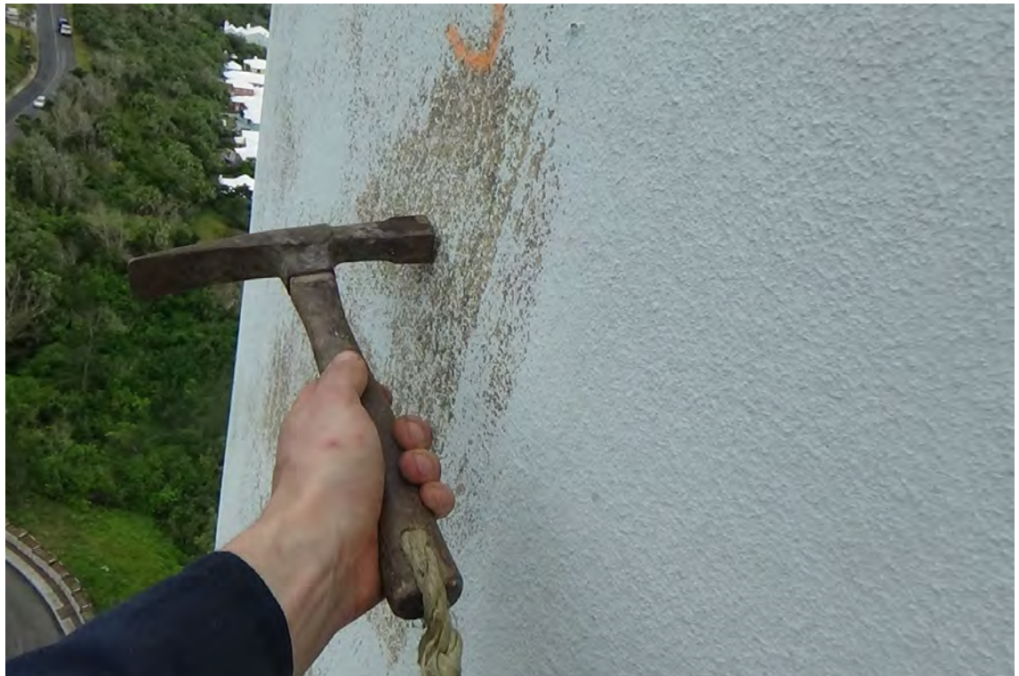
225' S—The concrete wall was hammer tested at various elevations to determine the composition and the hardness of the concrete. All the square footage which was observed and tested during the two exterior inspection drops, proved to be intact and solid.
