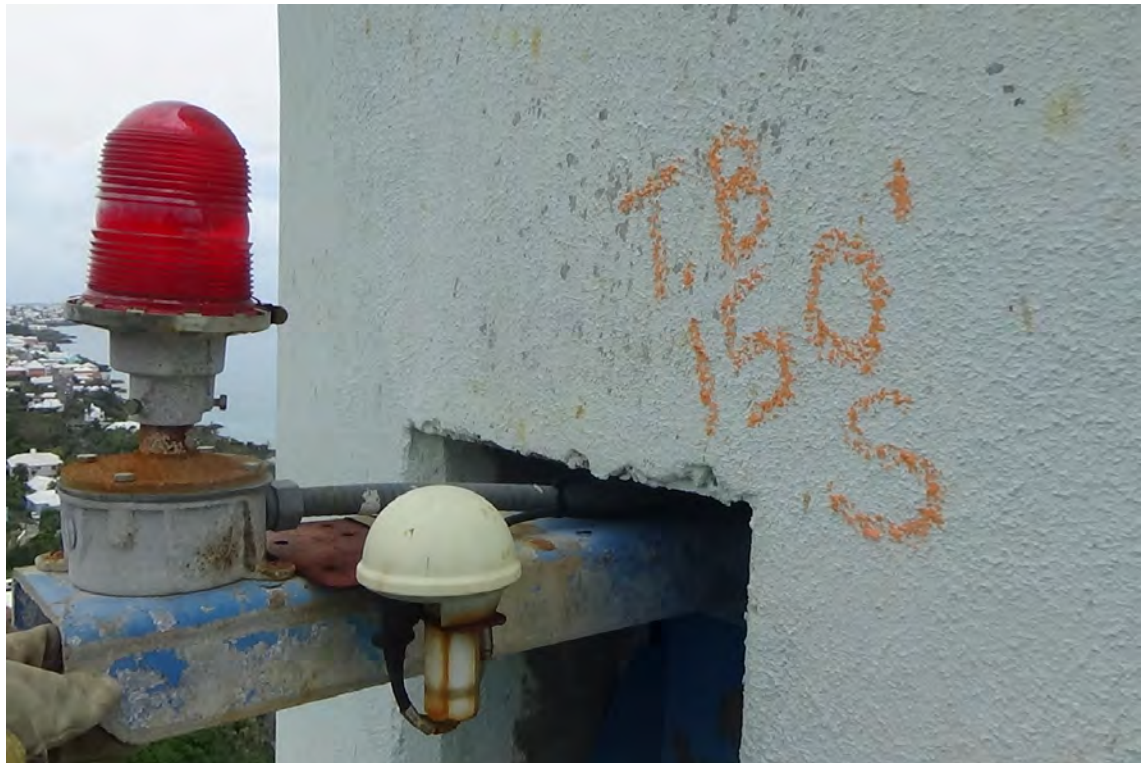
150' S—Aircraft obstruction light and components are all in satisfactory condition. The paint on the mounting bracket is badly worn.
