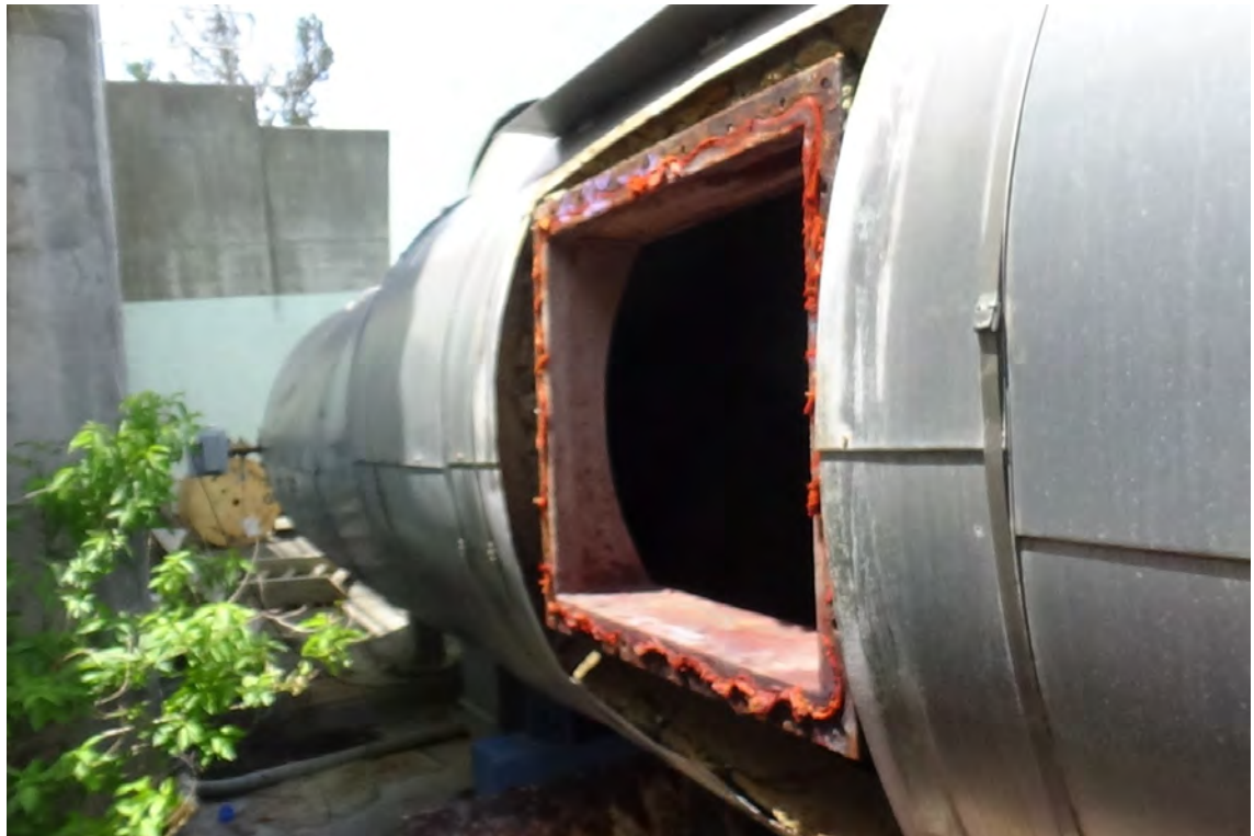
4' N/F1—The access door to flue #1 is located in the horizontal breaching duct approximately 30' from the base of the chimney. The opening measures 32" by 25". All the 1/2" bolts securing the access door were extremely corroded and were cut with a grinder/torch in order to remove the door.
