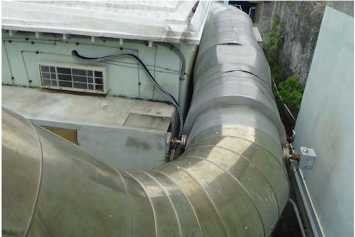
13' SE—View looking at the top of flue #1 ductwork displays no major damage or deficiencies. A small void can be seen on the top of flue duct where the two overlapping sections of cladding have separated exposing the insulation underneath.
