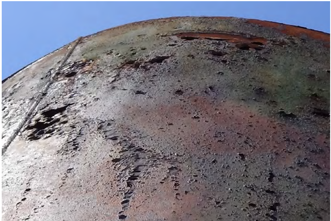
255' NE—More areas of corroded cladding at the top of flue #2. The void in the top right corner of the photo is near 8" in length. The horizontal weld attaching the rain cap to the cladding has cracked in this area. A small amount of overhang is visible which displays the misalignment between the components.
