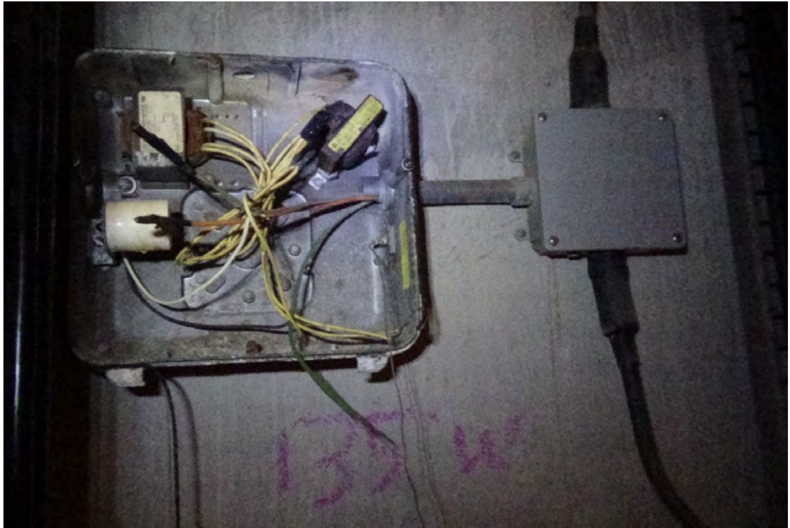
135' W—A single lighting fixture located at approximately 135' was found to be open with the cover and bulb removed. This light is located directly below the leak in the drain pipe. It is likely that moisture penetration into the unit has caused damage inside the light casing.
