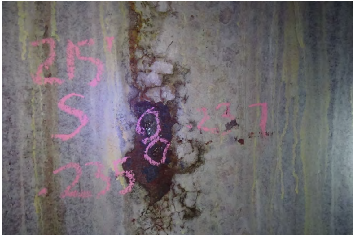
215' S/F1—A small area of scale was removed in order to take an ultrasonic measurement. Multiple layers of scale needed to be removed with a chipping hammer before measureable steel was found. Steel thickness measurements were found to be deteriorated but within acceptable ranges.
