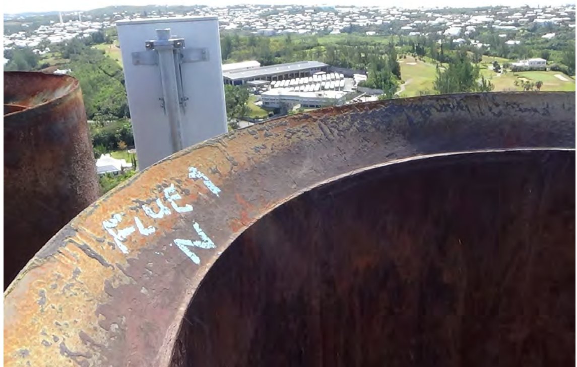
255' N—View looking at the top of flue #1 rain cap. The cap measures 6" in width and displays a moderate amount of deterioration throughout. The top of the liners were at one time painted. That may explain the blotchy appearance as the primer coat has mostly deteriorated.
