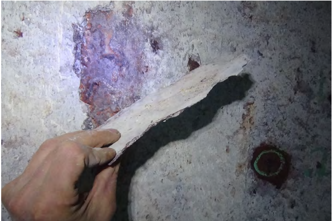
170' W/F2—Scaling is typical throughout the height of the liner. A piece of scale approximately 1/16" thick is displayed by the inspector. This was a common sight during both flue inspections.
