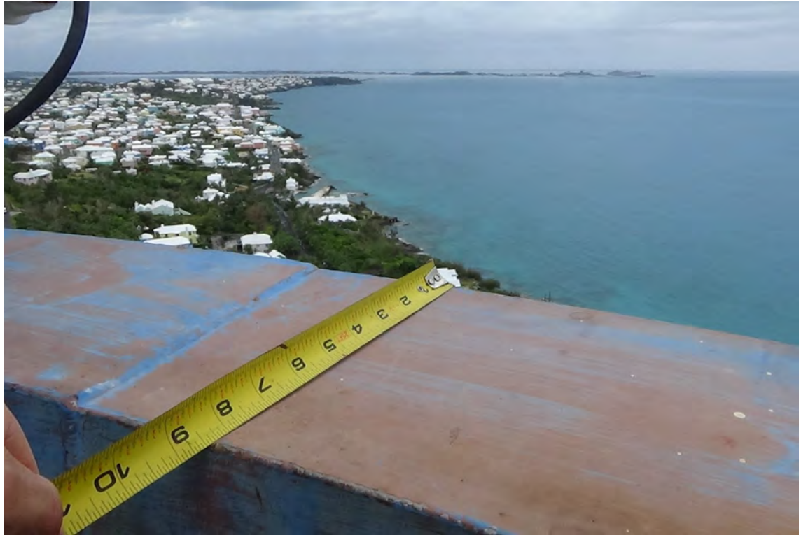
250' NW—The concrete rain cap measures 8 ½" in width. The top coat of blue paint appears weathered throughout the entire rain cap. The red primer is visible beneath the worn paint.
