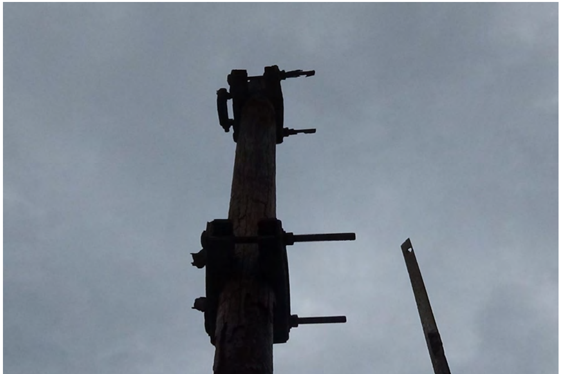
250' NW—An extreme amount of rust and scale are visible on the post and hardware of the obsolete, satellite transmitter mast.
