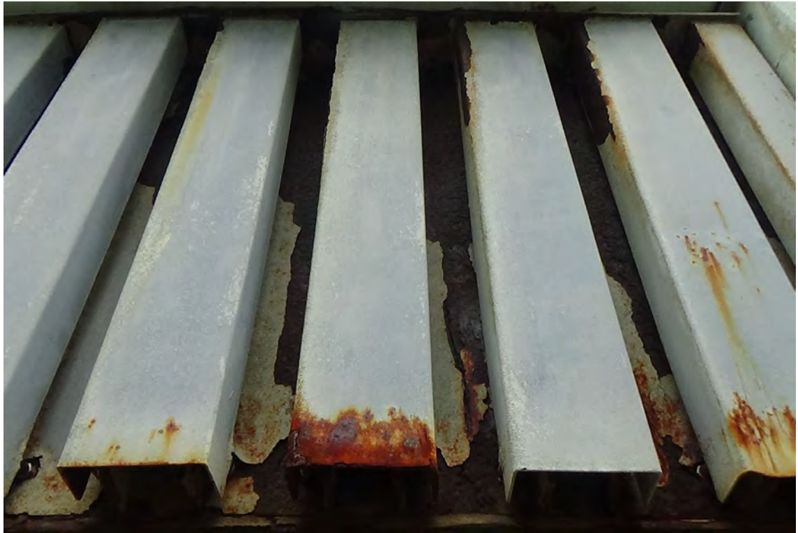
8' W—The vent covering over the annular space access door displays significant amounts of peeling paint, exposing rusted and pitted steel beneath. Corrosion holes are visible towards the bottom of the steel channels.
