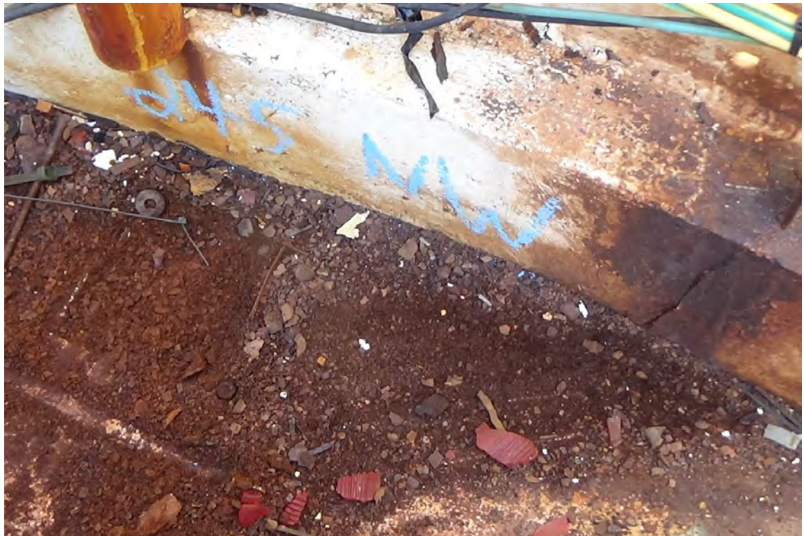
245' NW—An outline of the north west drain is visible on the left side of the photo. A fair amount of dirt and debris has settled in this area, clogging the drain pipe. The drain cover is depressed approximately ½" into the concrete creating a catch basin for debris.
