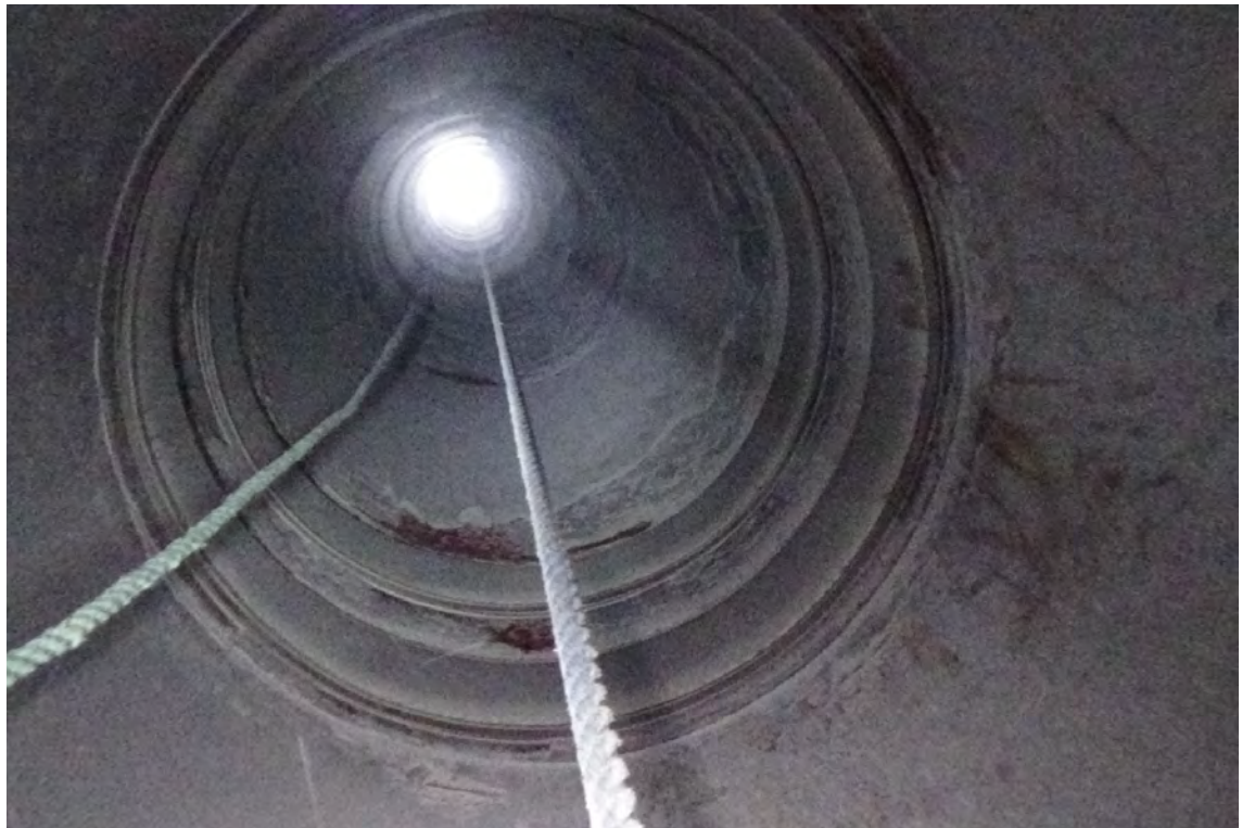
20' E/F1—View looking up the interior of flue #1 shows no signs of bulging or buckling within the liner wall. The expansion bellows system can be seen directly above.
