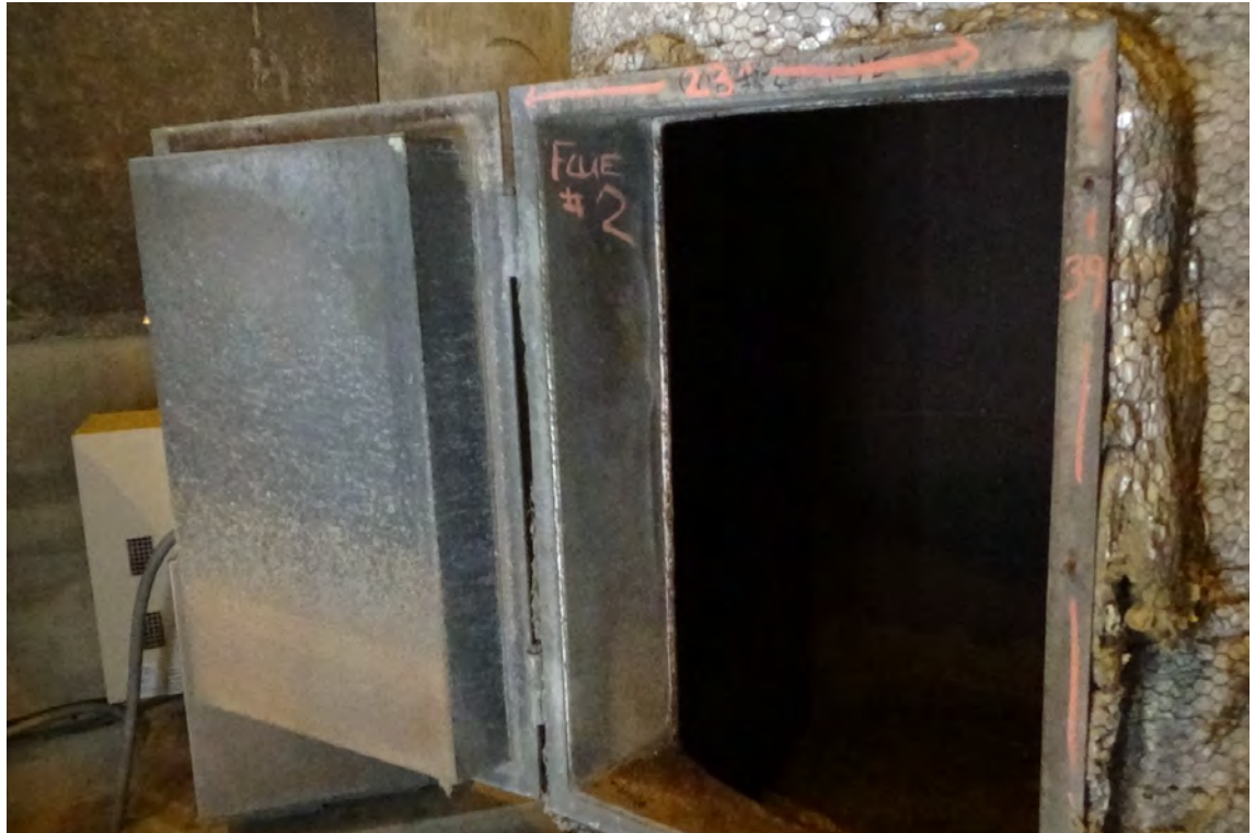
2' E/F2—The access door to the base of flue #2 measures 23" wide by 39" high. The door opens and closes freely. It is secured by three 3/8" bolts with wingnuts.
