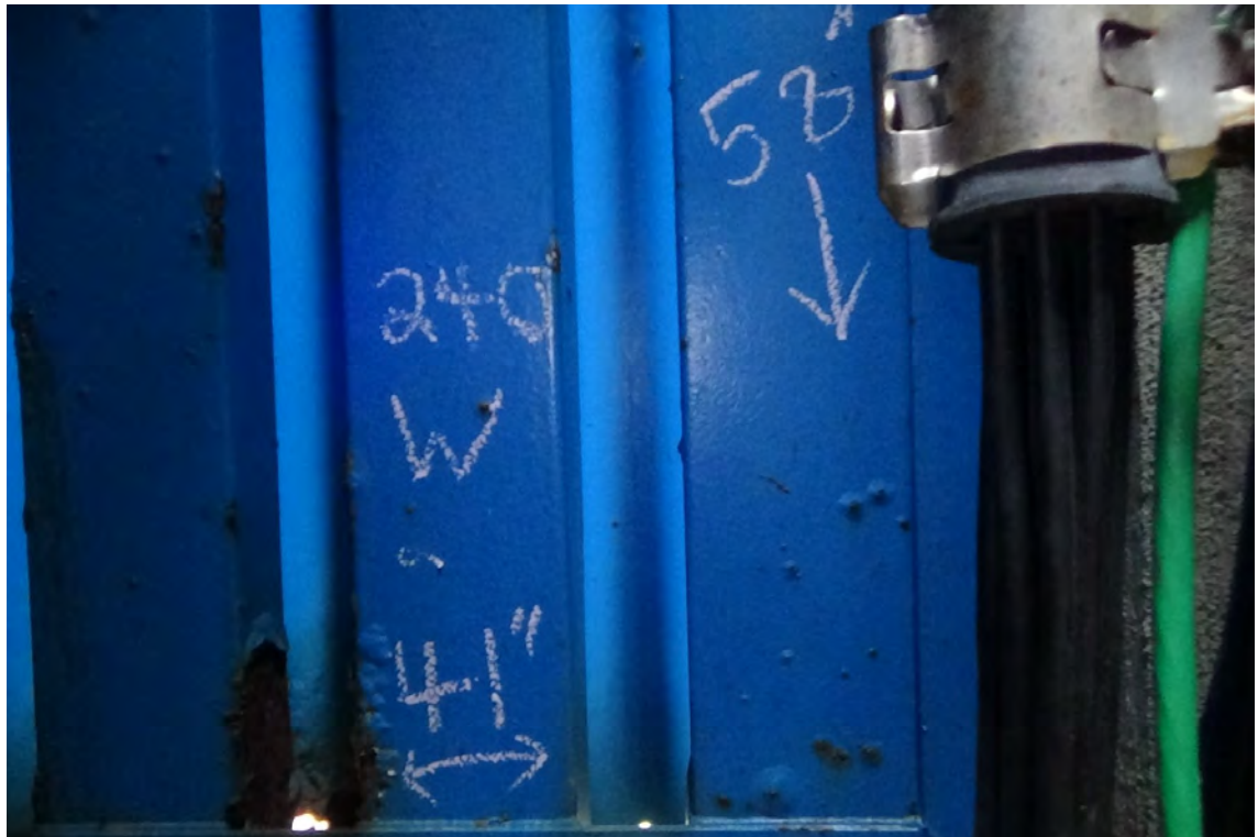
240' W—Field measurements of the vent cover are indicated. The blue paint is peeling towards the bottom of the channels due to rust and scale build-up.
