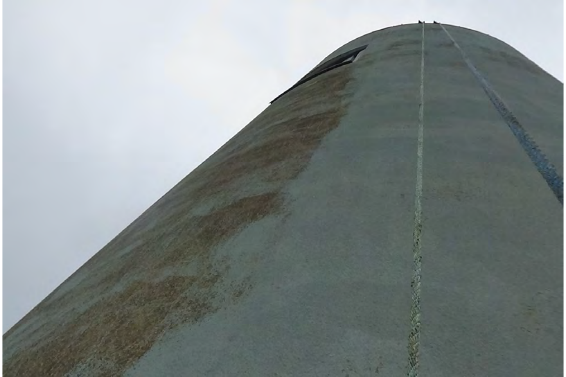
225' S—The protective coating directly beneath the annular vent has completely deteriorated for approximately 25'. The paint to the right of the vent displays a much more consistent finish.
