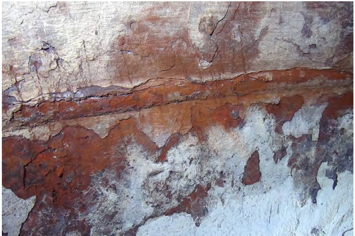
220' W/F2—Horizontal welds were cleaned and inspected at various elevations. The heavy scale had to first be removed in order to view the welds, which appeared rusted and pitted. However, they contained a consistent profile without signs of cracking.
