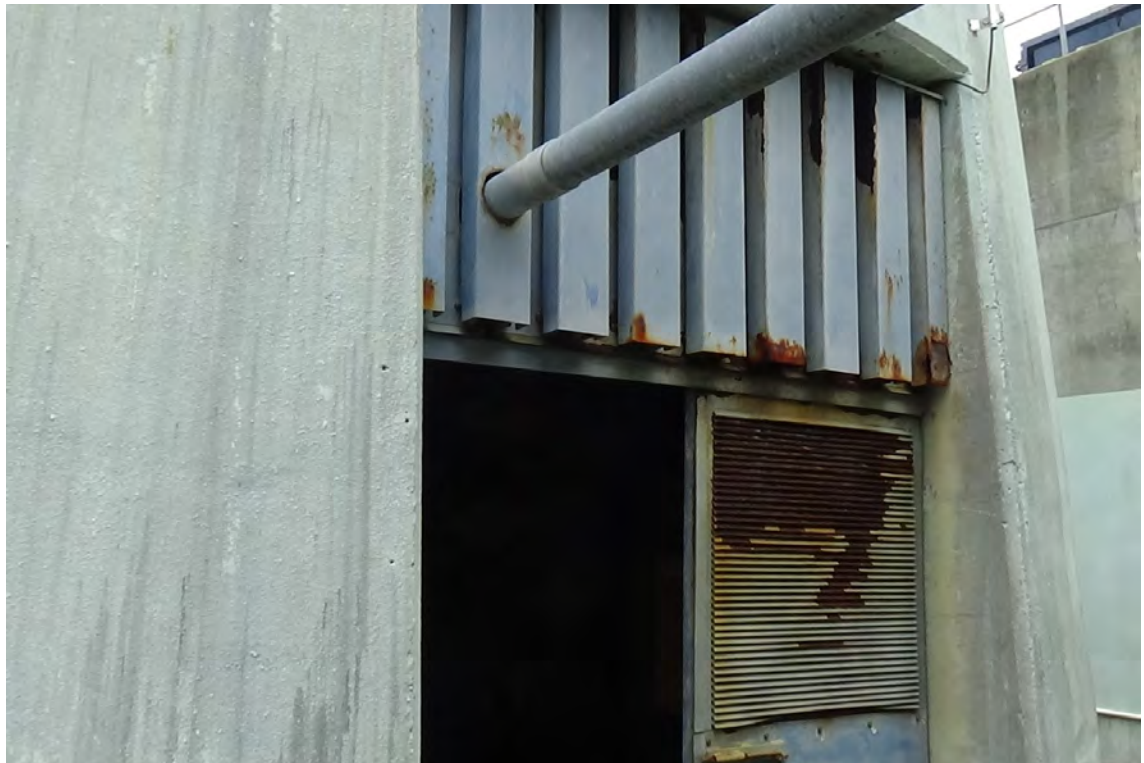
0' W—The two man doors providing access to the annular space were found to be in good working order. The blue paint over the vent portion of the doors is badly deteriorated, exposing significant rust and scale beneath.
