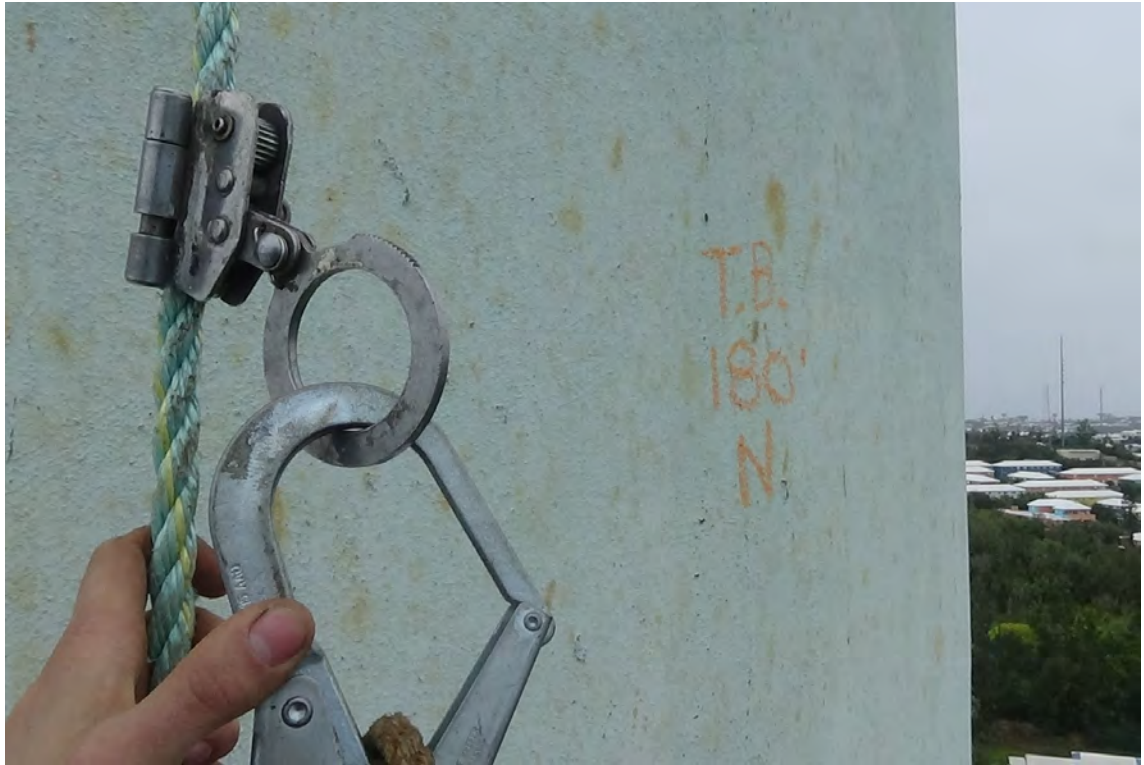
180' N—Below 200' a spotty brown staining is visible throughout the exterior coating. These stains can be attributed to steel scale being blown out the interior of the liners. The staining is more prominent on the north side of the column and diminishes as one descends towards the base.
