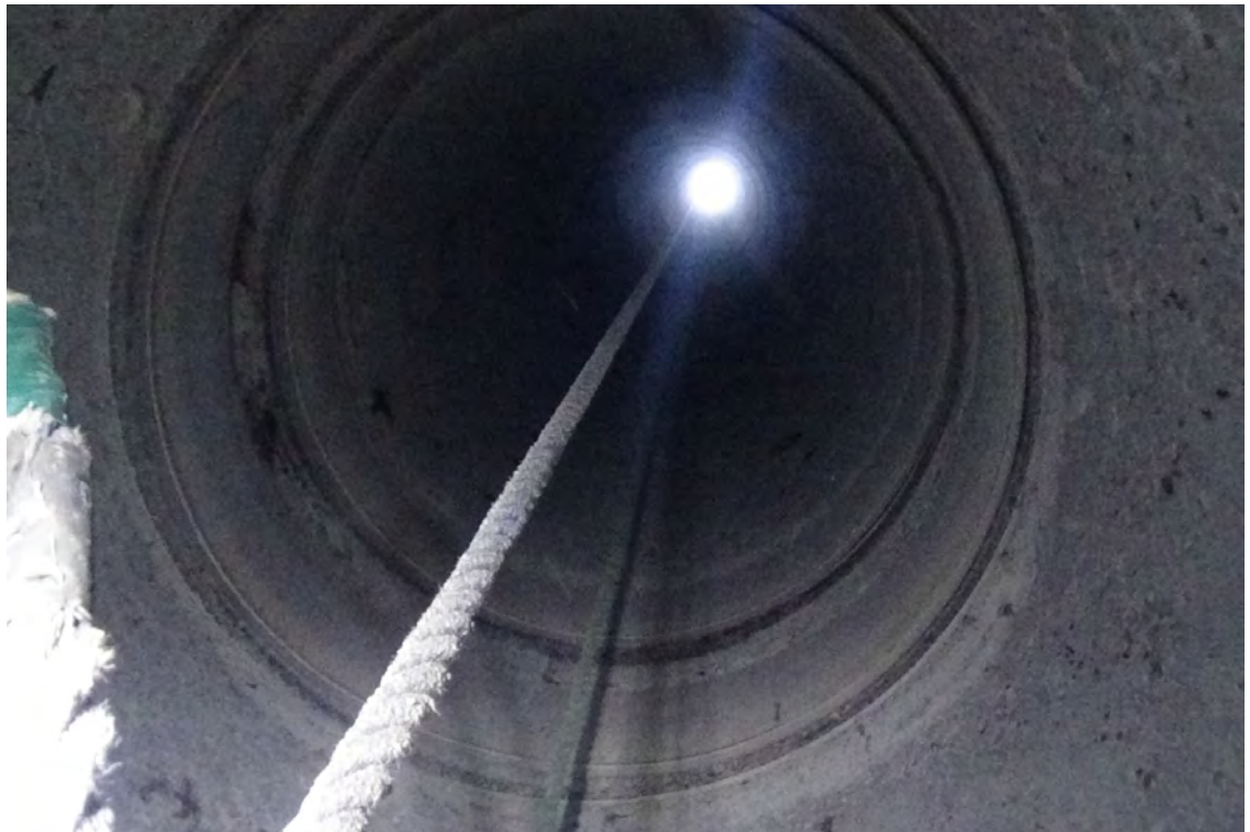
20' W/F2—View looking up the interior of flue #2 shows no signs of bulging or buckling within the liner wall. The expansion bellows system can be seen directly above.
