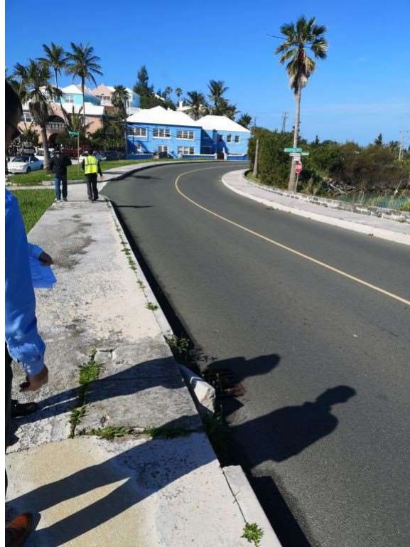
Figure 6: Broken kerb near west side of Bridge
