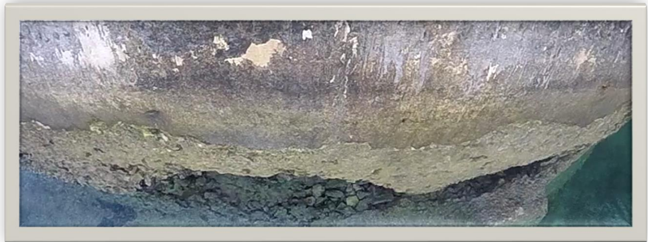
Figure 2: South Face view of South East edge of the landing showing erosion of the concrete from the bottom of landing above the footing to be repaired.
