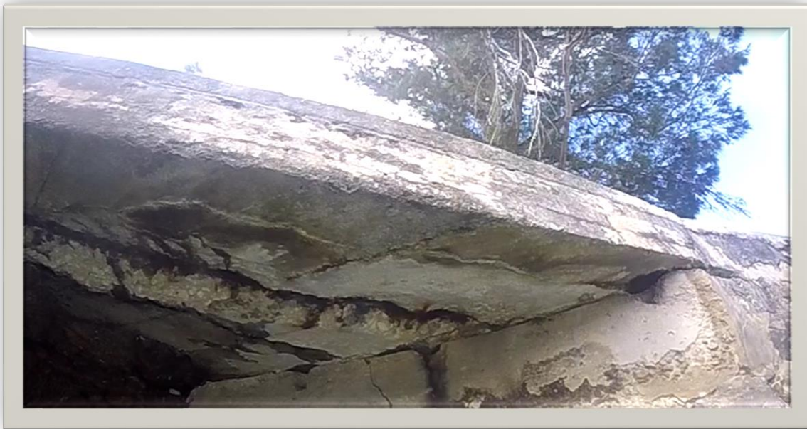
Figure 14: South Face view of exposed reinforcement bars and cracking in the wall.
