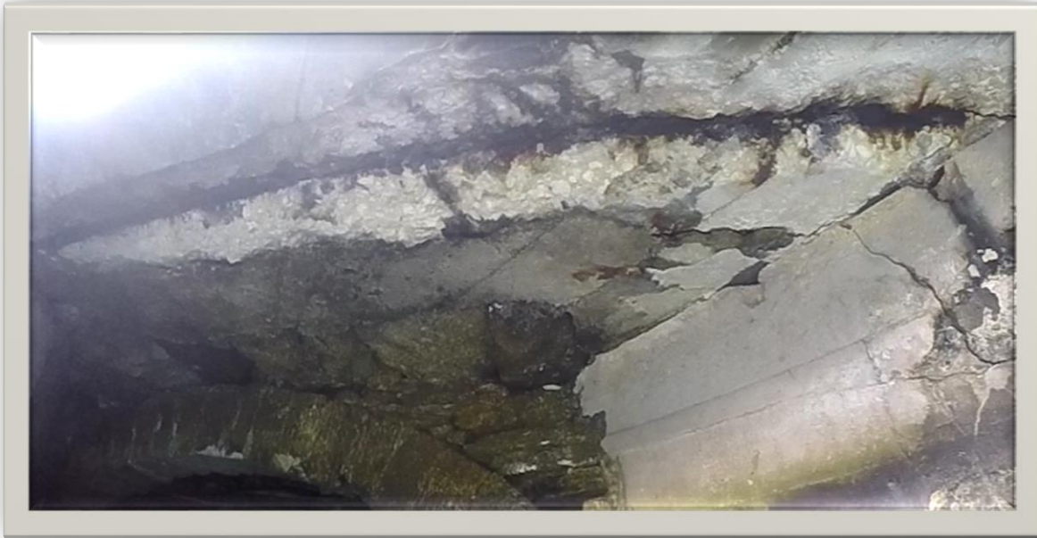
Figure 13: Exposed rebar above archway.
