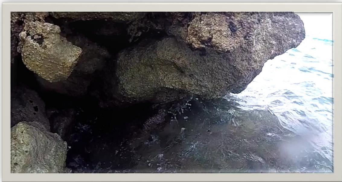
Figure 24: Cavity on Eastern Face of Landing.
