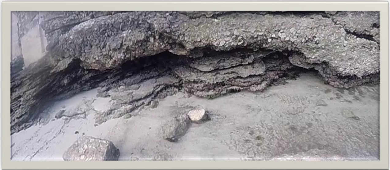
Figure 7: South Face showing undermining of the concrete slab.
