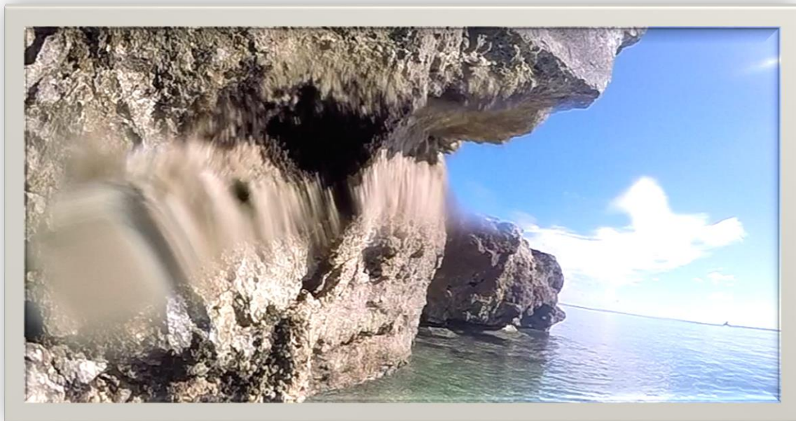
Figure 4: Eastern Face showing erosion of concrete below front edge of landing.
