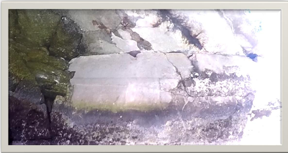
Figure 13: South Face view of crack on the East wall of archway.
