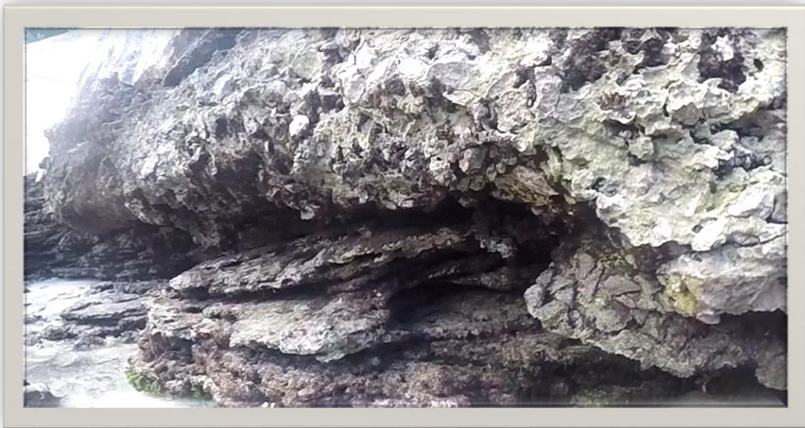
Figure 8: South Face enhanced view of undermining.
