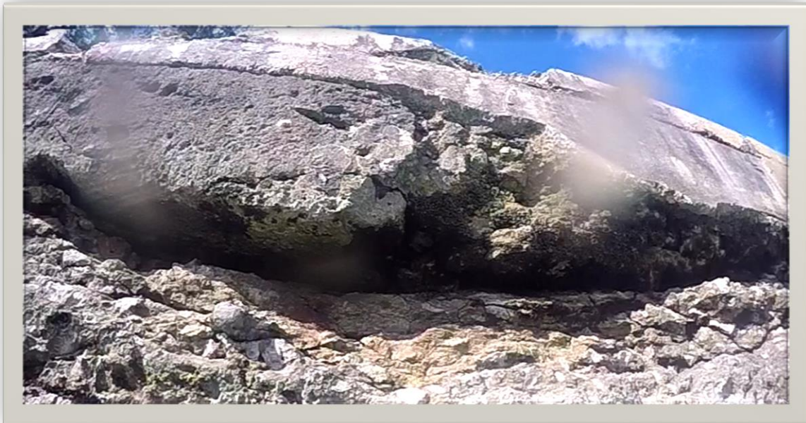
Figure 14: South Face showing crack below the top concrete slab.
