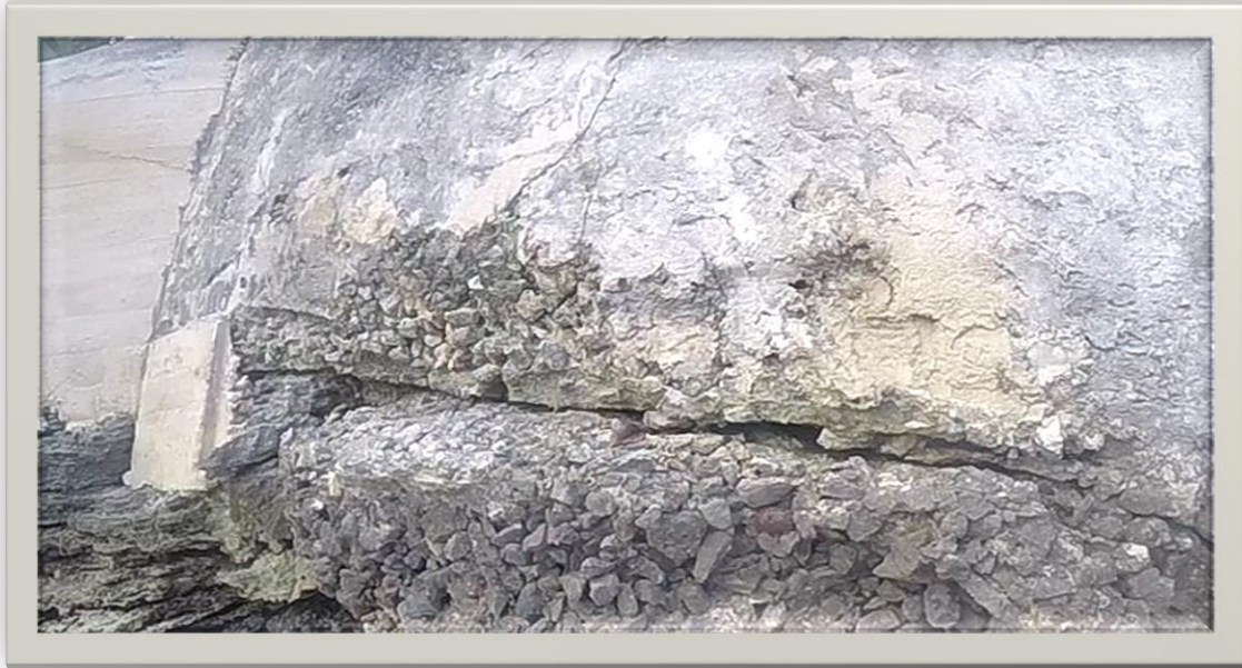
Figure 9: South Face showing a horizontal crack in the concrete slab and exposed aggregate.
