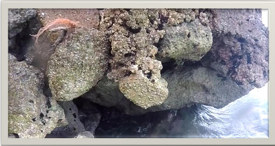
Figure 17: Typical erosion of concrete.
