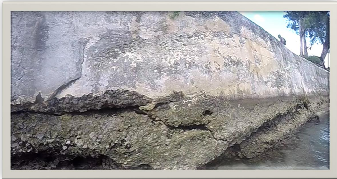
Figure 10: South Face showing exposed base of landing with horizontal cracking and undermining.
