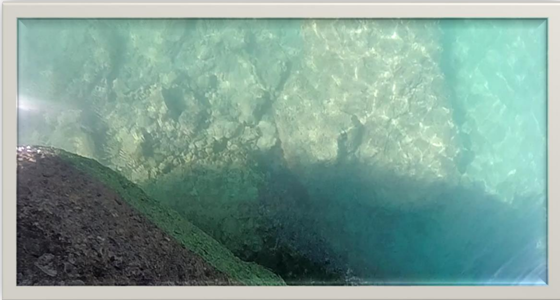
Figure 3: Boulder and rubble in water to be removed from East end of landing.
