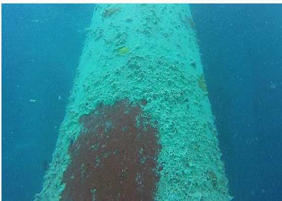
Fig. 3w - 2 nd Level 2 inspection, H-BD3, minimal corrosion of pile
