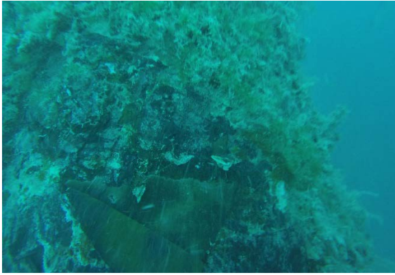
Fig. 3s - Protective coating peeling away on H-BD2, minimal corrosion
