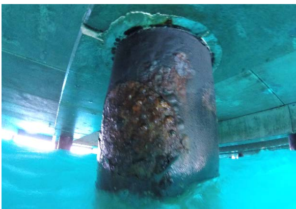
Fig. 1t - Typical example of corrosion of exposed steel in splash zone
