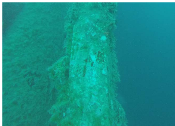
Fig. 3v - Level 2 inspection on anode, H-BD3
