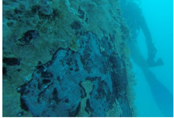
Fig. 3z - Level 2 inspection at base, H-MD2 – surface pitting and corrosion
