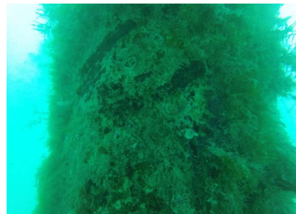
Fig. 2d 3 rd Level 2 inspection, Pile 165, protective layer not present
