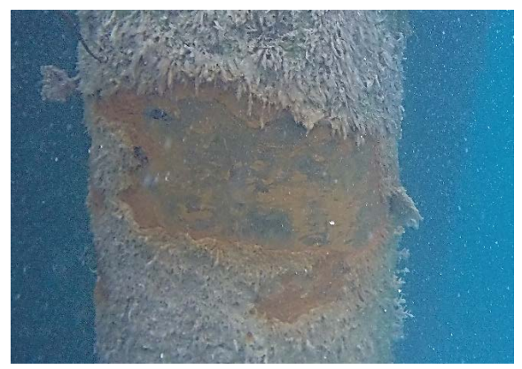
Fig. 3hh - Band of extreme corrosion, H-MD2
