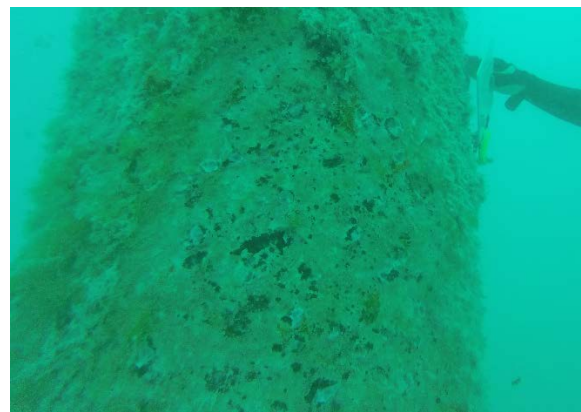
Fig. 3x - Level 2 inspection at base, H-BD1, no protective layer present
