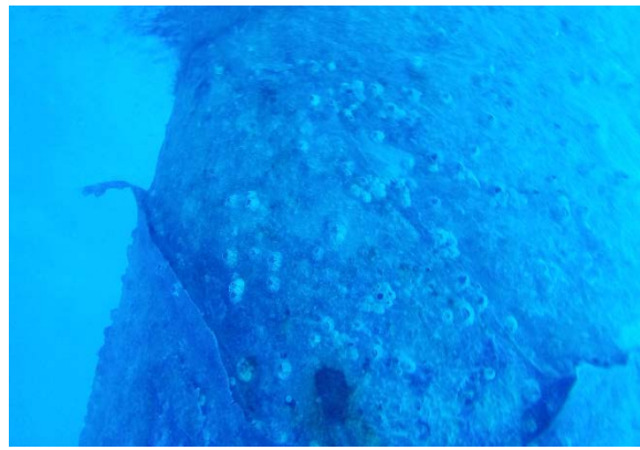
Fig. 1s - Protective coating peeled away just below surface
