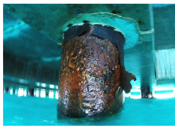
Fig. 1u Compromised protective coating and corrosion
