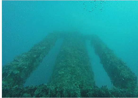
Fig. 3h - Anode on walkway dolphin
