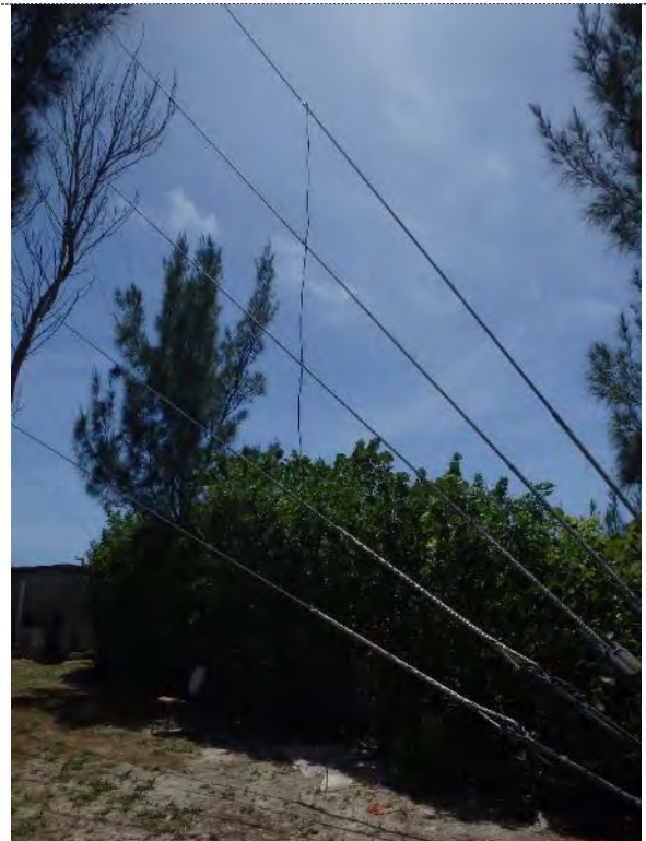
Anchor A grounding Photo File 272
