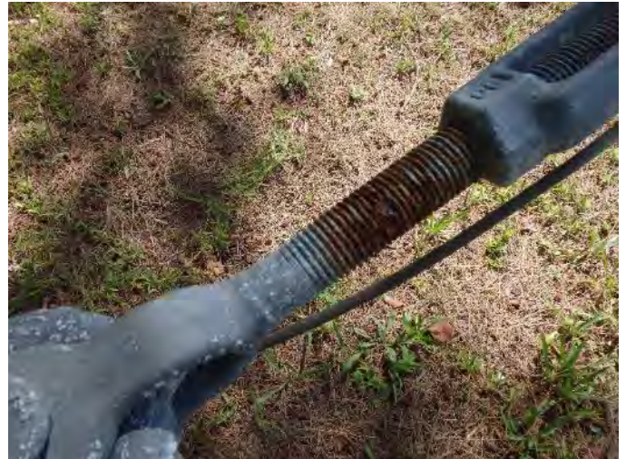
Anchor B hardware corrosion Photo File 294
