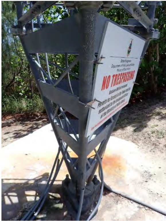
Tower base A leg Photo File 9
