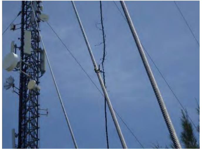
A 4 disconnected ground wire Photo File 286
