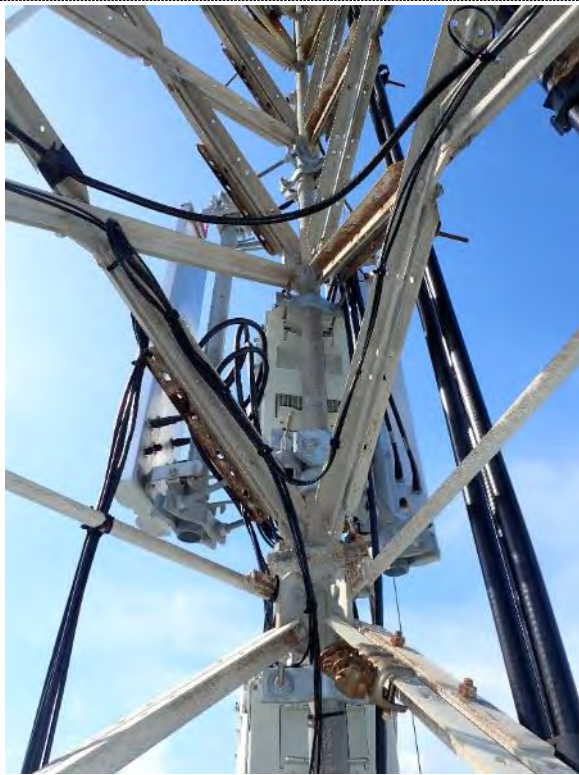
Radio #70, antennas #72, #73 Photo File 181
