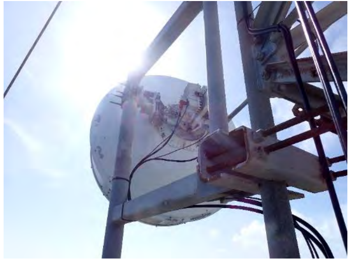
Antenna #62, radios #63, #64 Photo File 174
