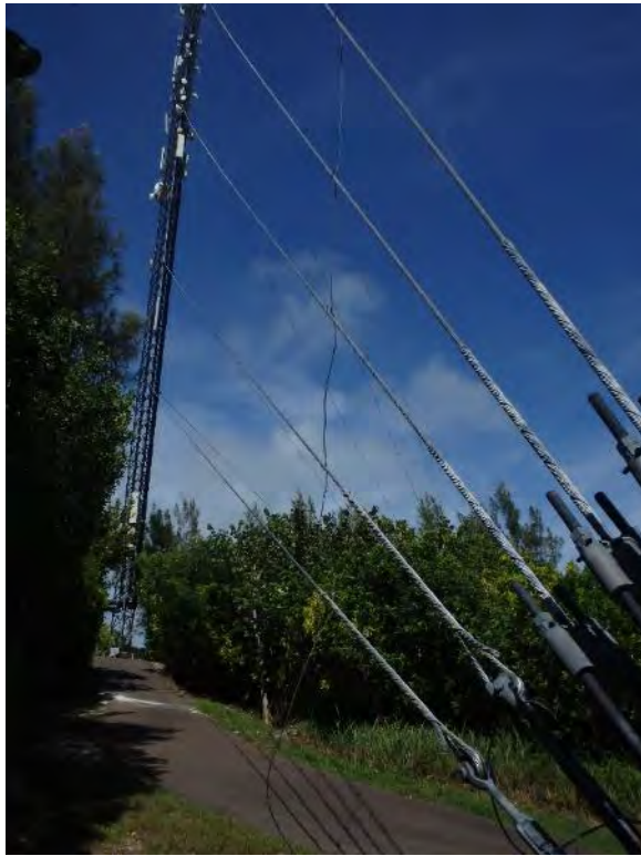
Anchor C grounding Photo File 321
