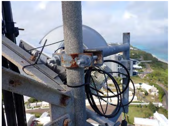
Antenna #75, radios #76, #77 Photo File 208
