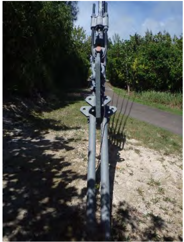
Anchor C fan plate out of alignment Photo File 326
