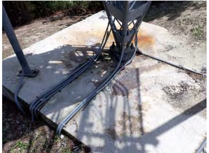
Tower grounding Photo File 18
