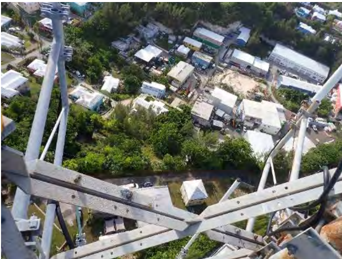
Horizontal missing from top of tower Photo File 259
