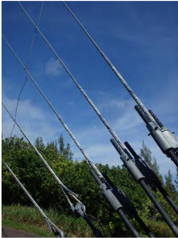
Anchor C missing end sleeves Photo File 325
