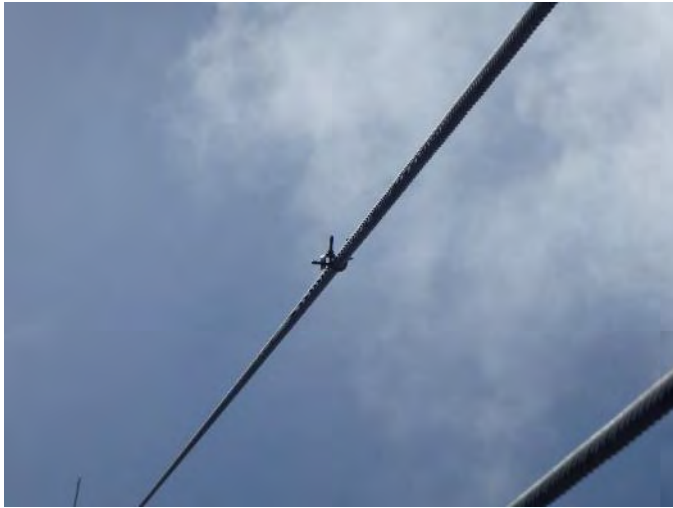
B 5 disconnected ground Photo File 301
