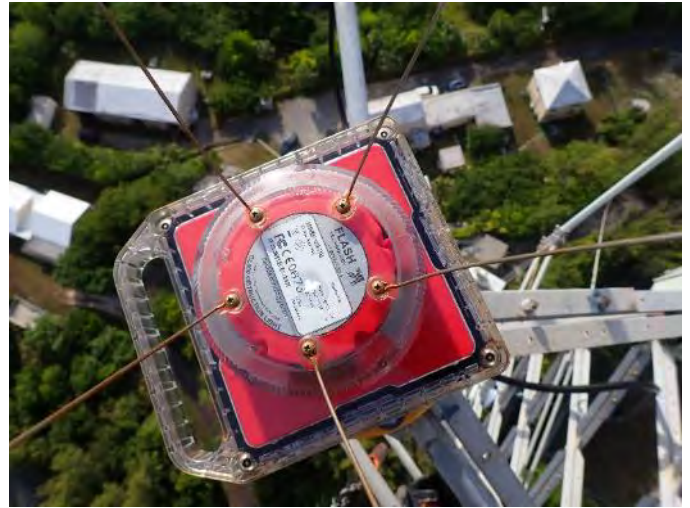
Operational beacon Photo File 262
