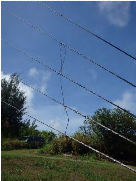
Anchor B grounding Photo File 299
