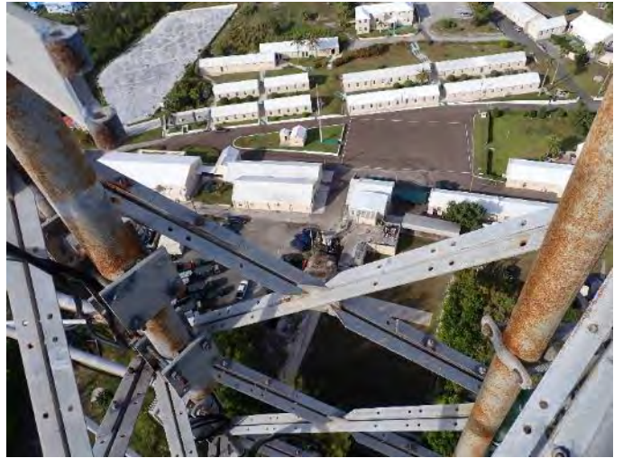
Horizontal missing from top of tower Photo File 258
