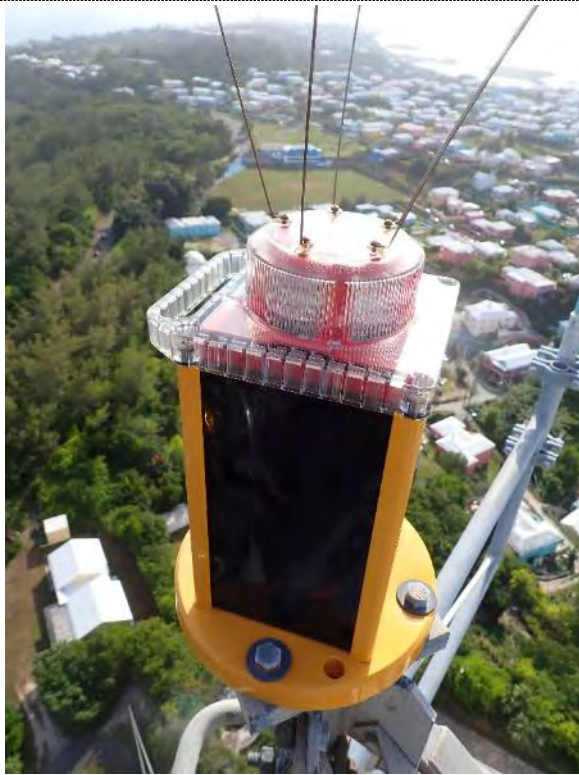
Operation beacon Photo File 261
