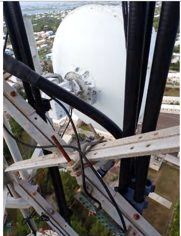
Stiff arm attached to tower diagonal Photo File 228
