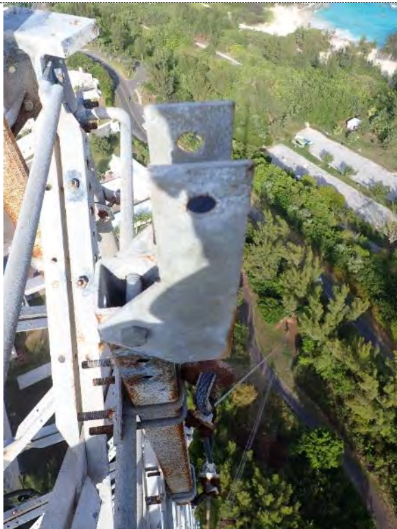
Top safety cable bracket Photo File 263
