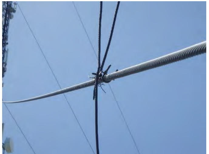
B 5 disconnected ground Photo File 300
