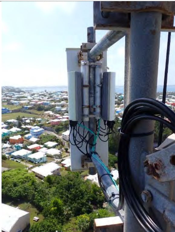
Antenna #37, radios #38, #39 Photo File 139
