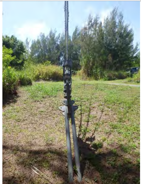
Anchor B fan plate out of alignment Photo File 312
