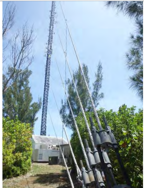
Anchor A grounding Photo File 284
