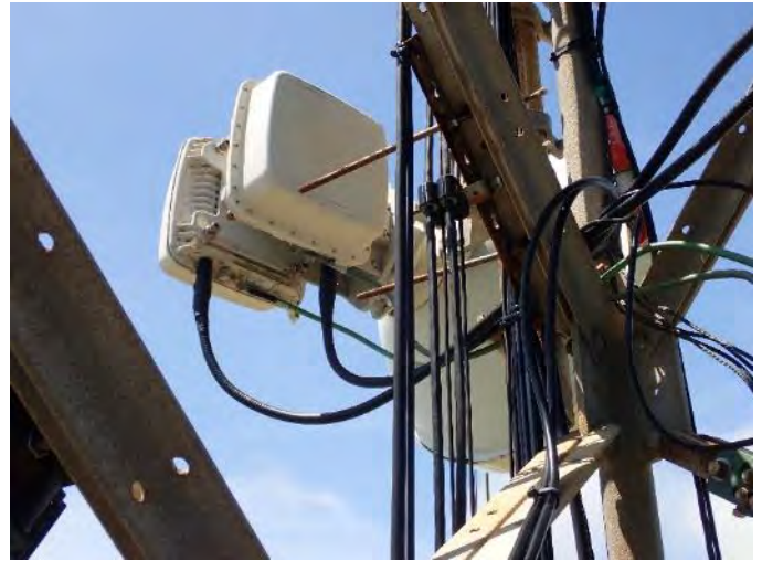
Antenna #12, radios #13, #14 Photo File 90
