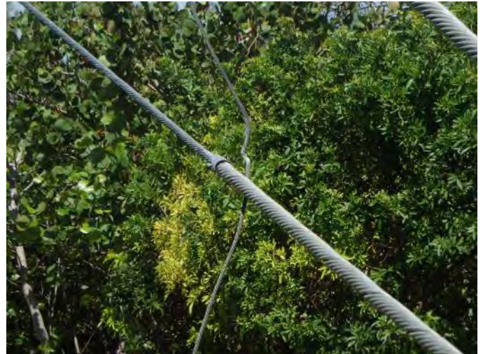
C 1 missing ground clamp Photo File 322
