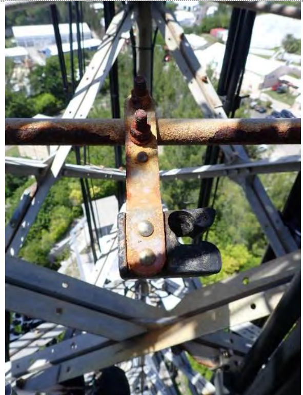
Safety cable keeper condition Photo File 72
