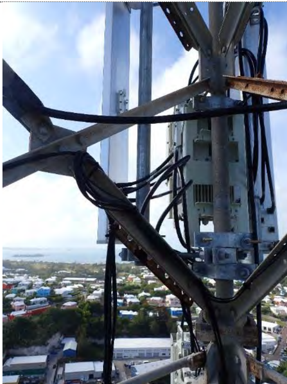
Radio #70, antennas #72, #73 Photo File 195
