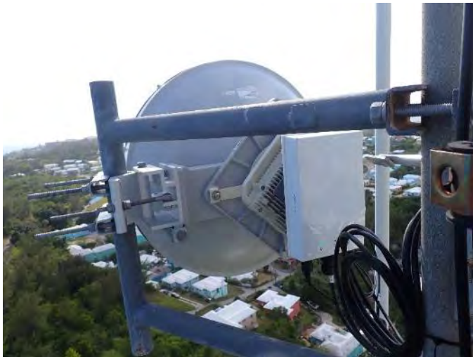
Antenna #78, radios #79, #80 Photo File 209
