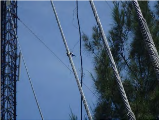
A 3 disconnected ground wire Photo File 285
