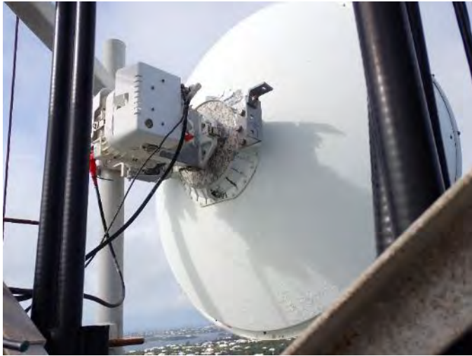
Antenna #87, radios #88, #89 Photo File 227
