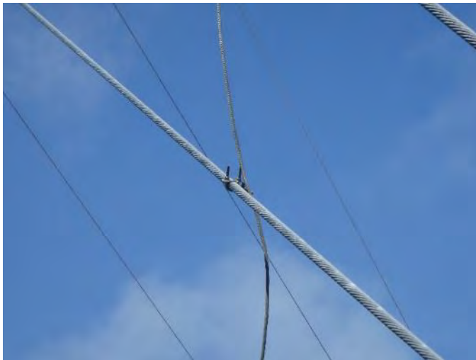
C 3 disconnected ground Photo File 323
