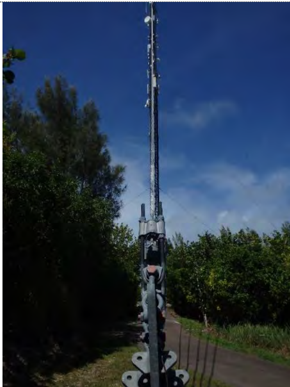
Anchor C fan plate out of alignment Photo File 327
